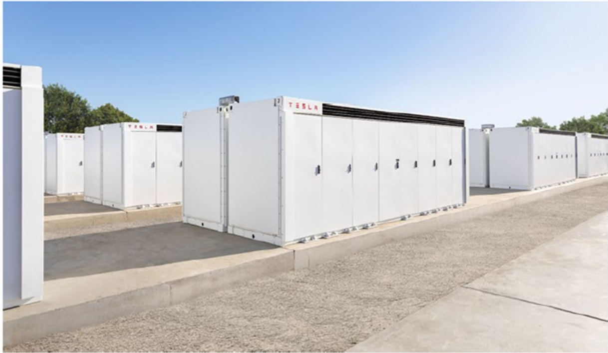
Figure 3-3: A typical BESS site
