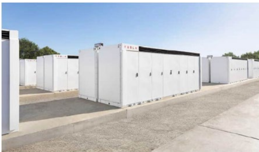
Figure 2-2 Tesla Megapak units (source: Ausgrid)
