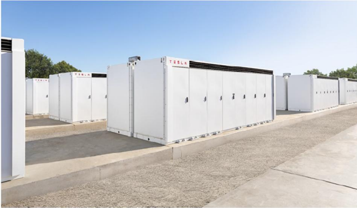
Plate 1: Example of a MegaPack 2XL containerised BESS arrangement
