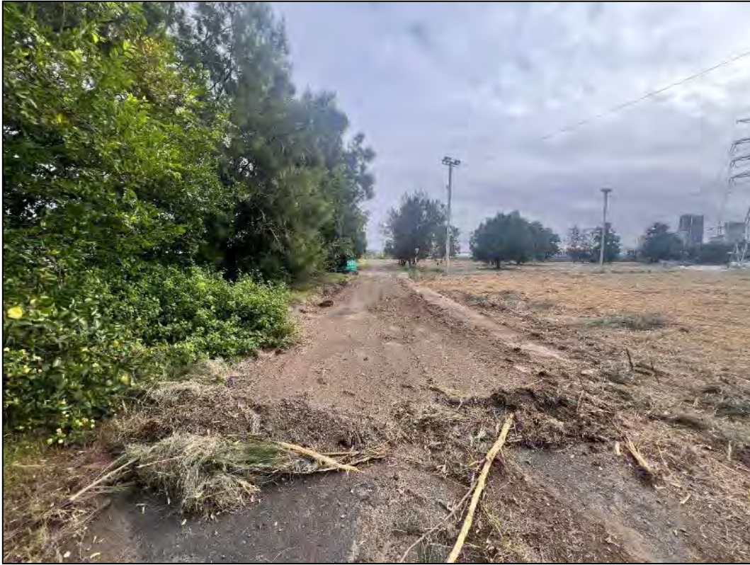
Plate 6: Further site disturbance and vegetation clearing along the southern boundary of the site.
