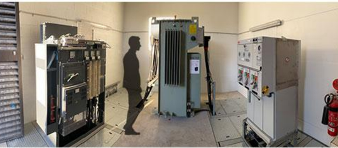
Inside a chamber substation
