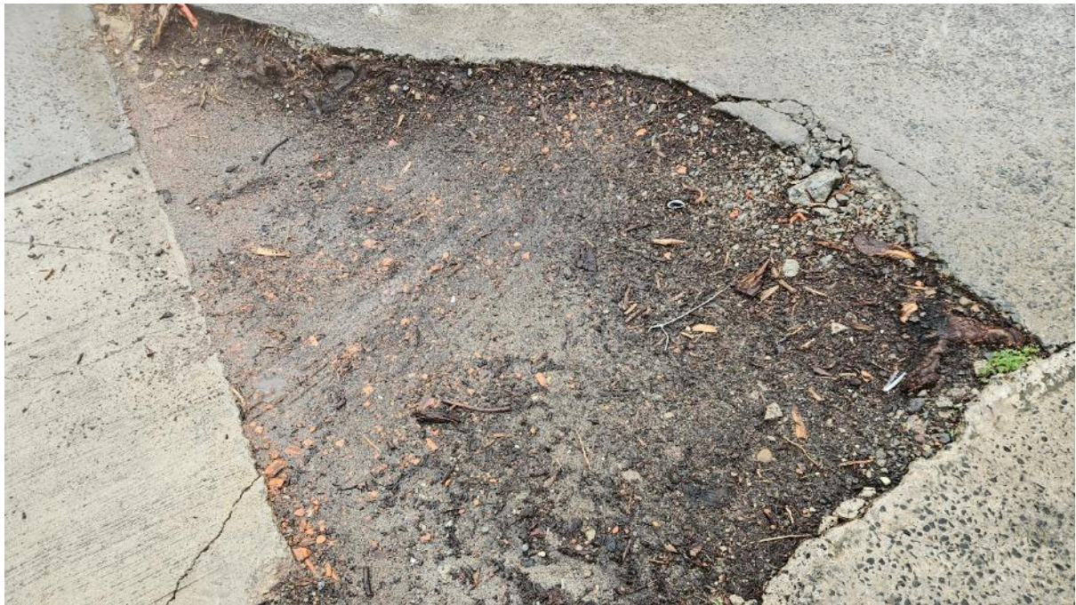
Plate 5. The damaged driveway showing dark sandy fill. (Source: Heritage Now 2025)
