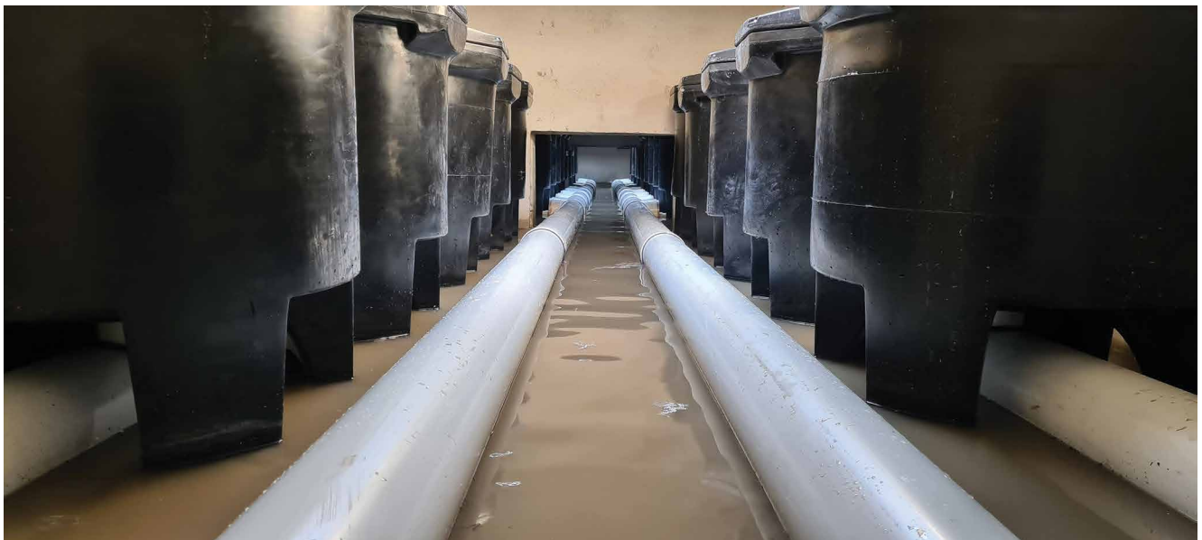
Figure 1 - AtlanFilters in a concrete chamber / vault
