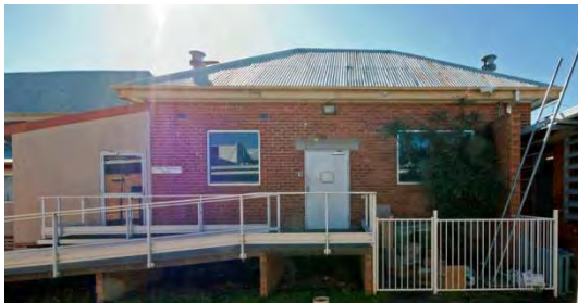
Figure 35 Significant reworking is evident on the south facade. The lintel to the left has been shortened by later brick changes, while the lintel to the right is completely missing perhaps due to the much larger window introduced. The only section of verandah surviving is on the left side of the image – Adaptive Architects Pty Ltd 2014
