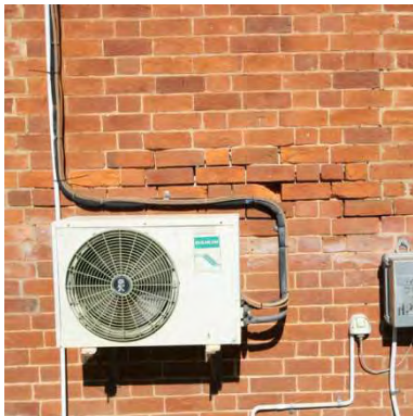
Figure 107 c1890 external wall where the soft bricks are being seriously damaged by air conditioning unit – the units need to be removed
