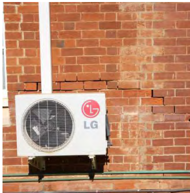
Figure 108 c1890 external wall at junction with 1926 addition where the stronger bricks are not suffering as greatly.
