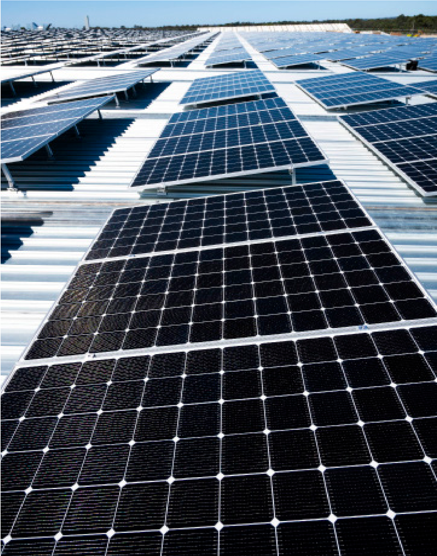
FIGURE 3.16 - Solar Panels installed at Development East Warehouse 1.
