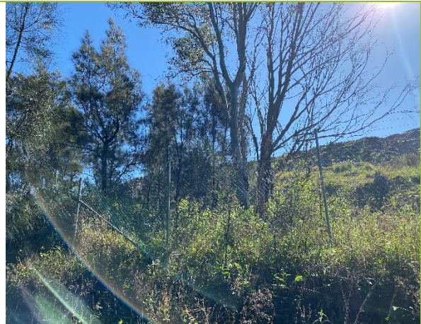
Photo plate 2: example of modified landform to east of Photo plate 1 (where construction of road embankment encroach into riparian zone).
