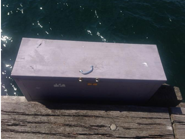
Figure 9 - Damaged Life Buoy Storage Unit at Walsh Bay
