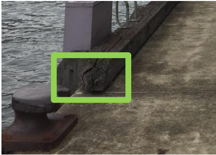
Figure 10 - Distance of Kerb in close Proximity to Pier Edge
