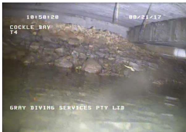
Figure 65: Seawall at the end of Transect 4 showing current PVC drainage pipe on left hand side. (Cockle Bay 170821 T4, 7:13)
