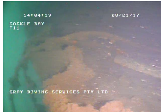
Figure 97: Silt behind the sheet piling (to the right of image) and drop in front of the sheet piling. (Cockle Bay 170821 T11, 4:16)
