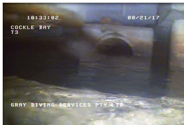
Figure 63: Storm water drain viewed over the top of the diffuser. (Cockle Bay 170821 T3, 5:54)
