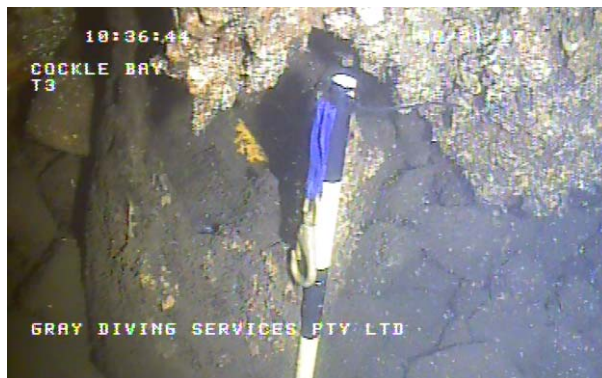
Figure 64: Degraded timber pile stump below concrete pour, against southern wall of storm water drain. Scale in 100 mm increments. (Cockle Bay 170821 T3, 9:19)
