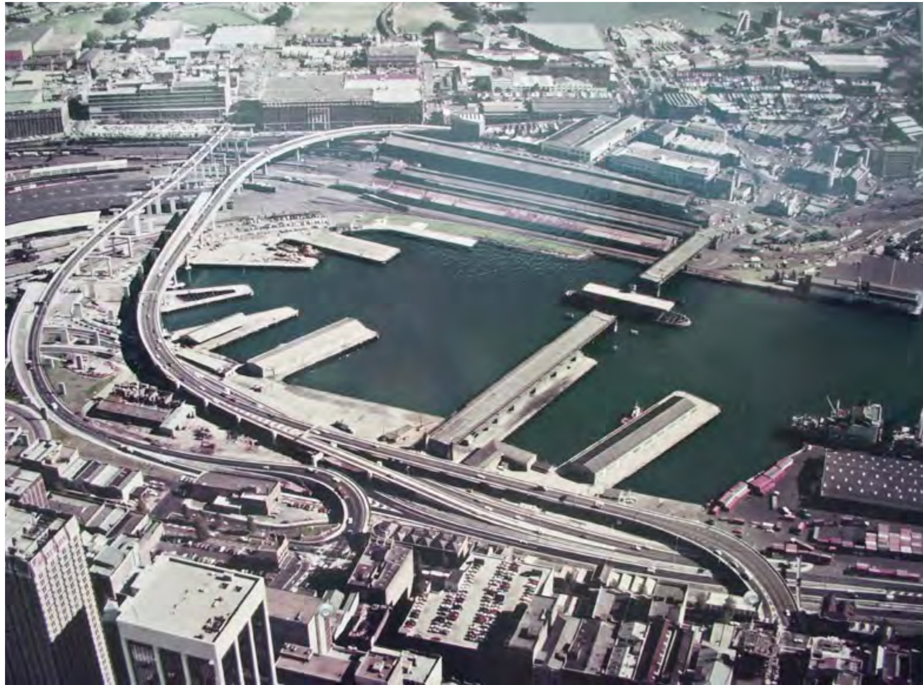
Fig. 18. Construction of Western Distributor during the 1980s showing the disruption to the direct route from Market Street to Pyrmont Bridge
