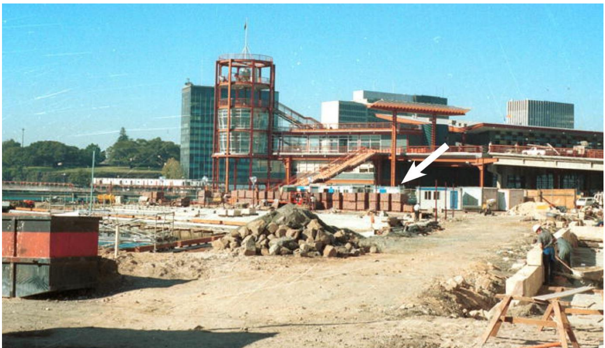
Figure 7.7 Looking southwest towards the subject site (white arrow) showing works associated with the building upgrade—the white framework in the background is for the existing steps situated outside the northern edge of the study area, June 1987. (Source: City of Sydney Archives, CRS 422/3/523 with GML overlay)
