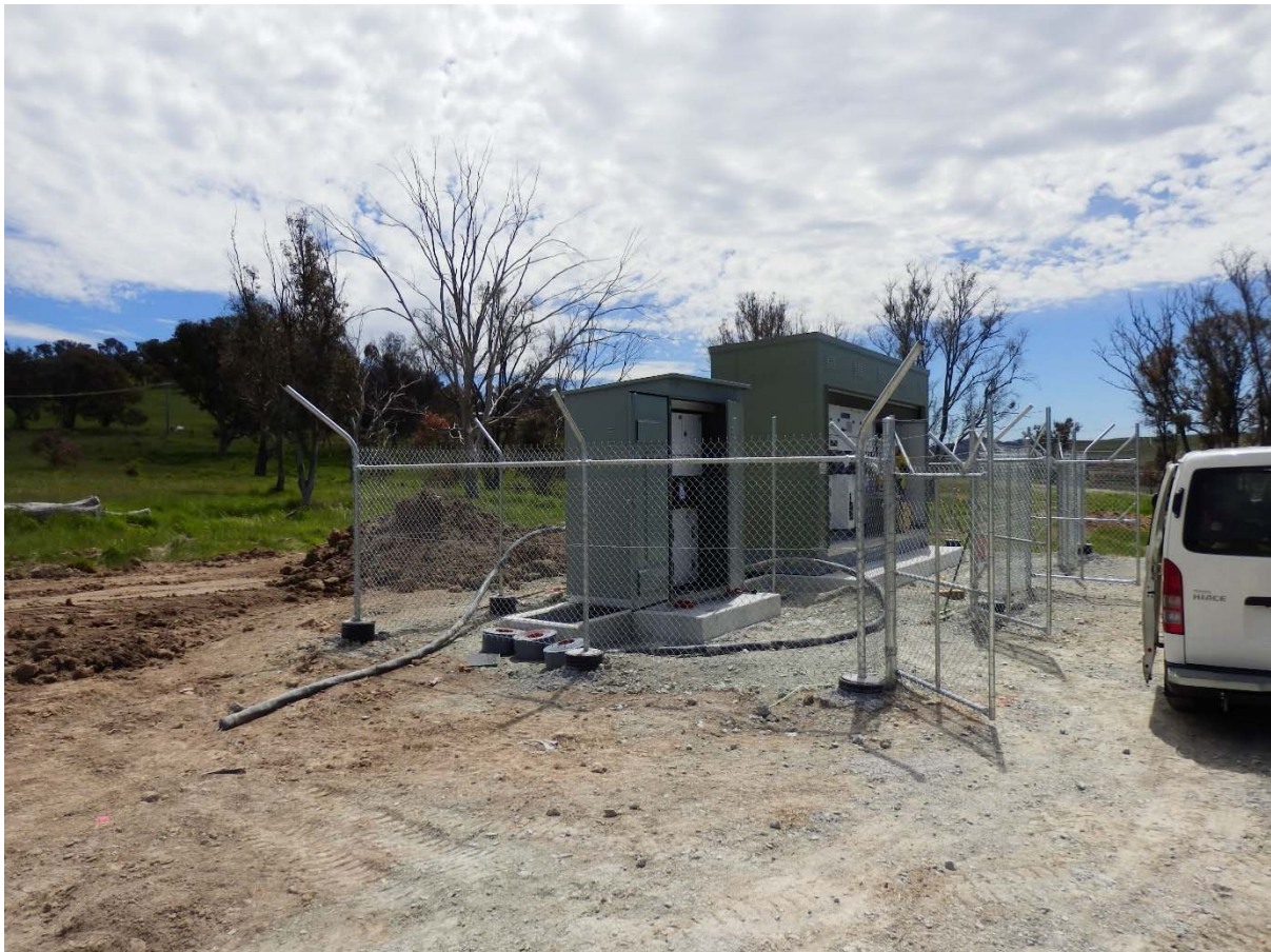
Figure 3-12 Example of a substation on delivery
