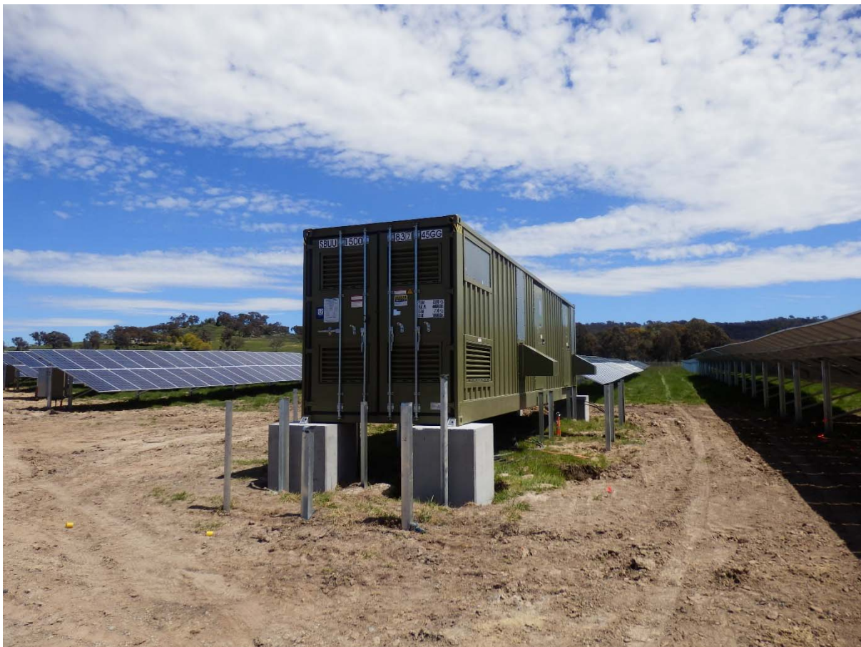
Figure 3-10 Example of a PV Box
