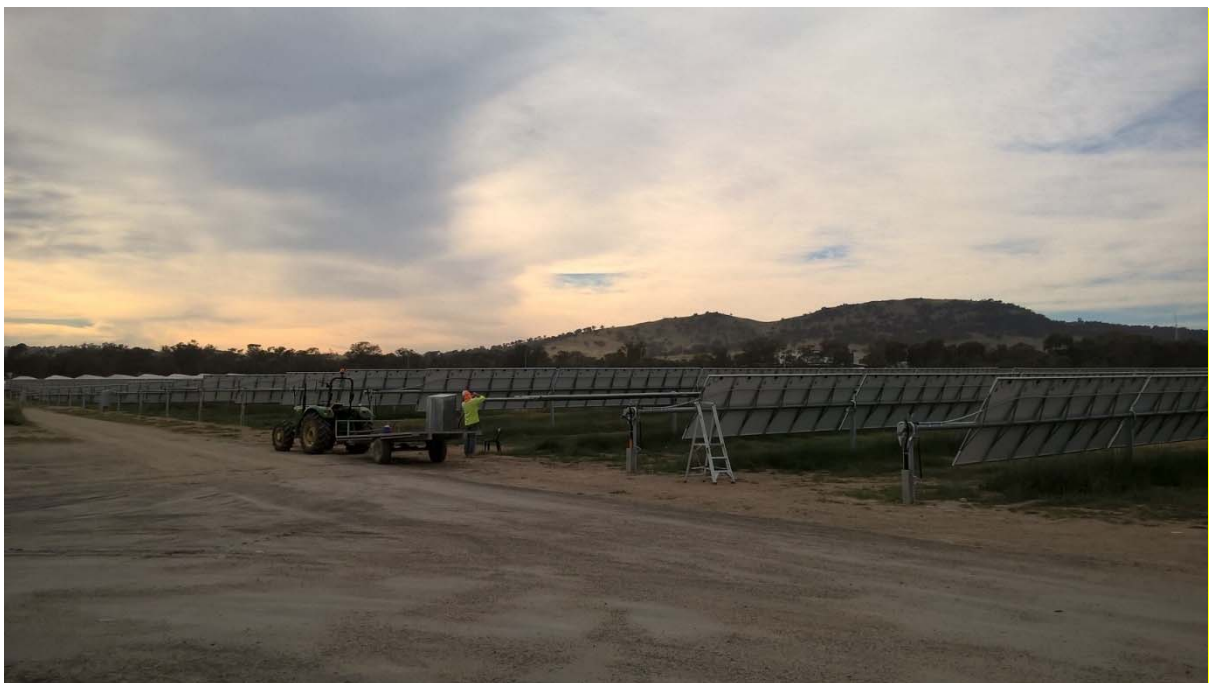
Figure 3-9 Example of solar arrays at Mugga Lane Solar Park
