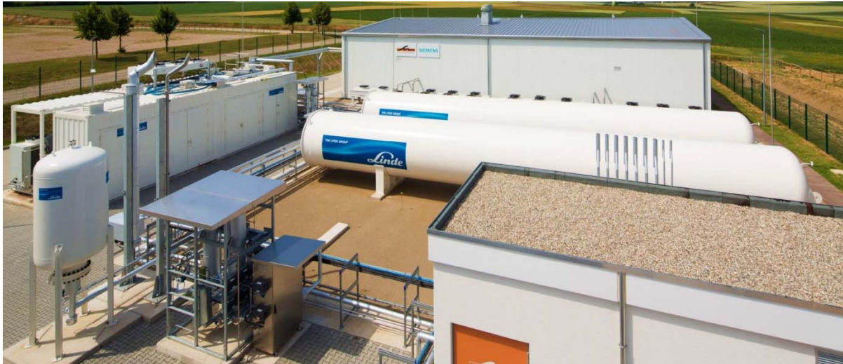
Figure 3-14 Example of Hydrogen Fuel Cell
