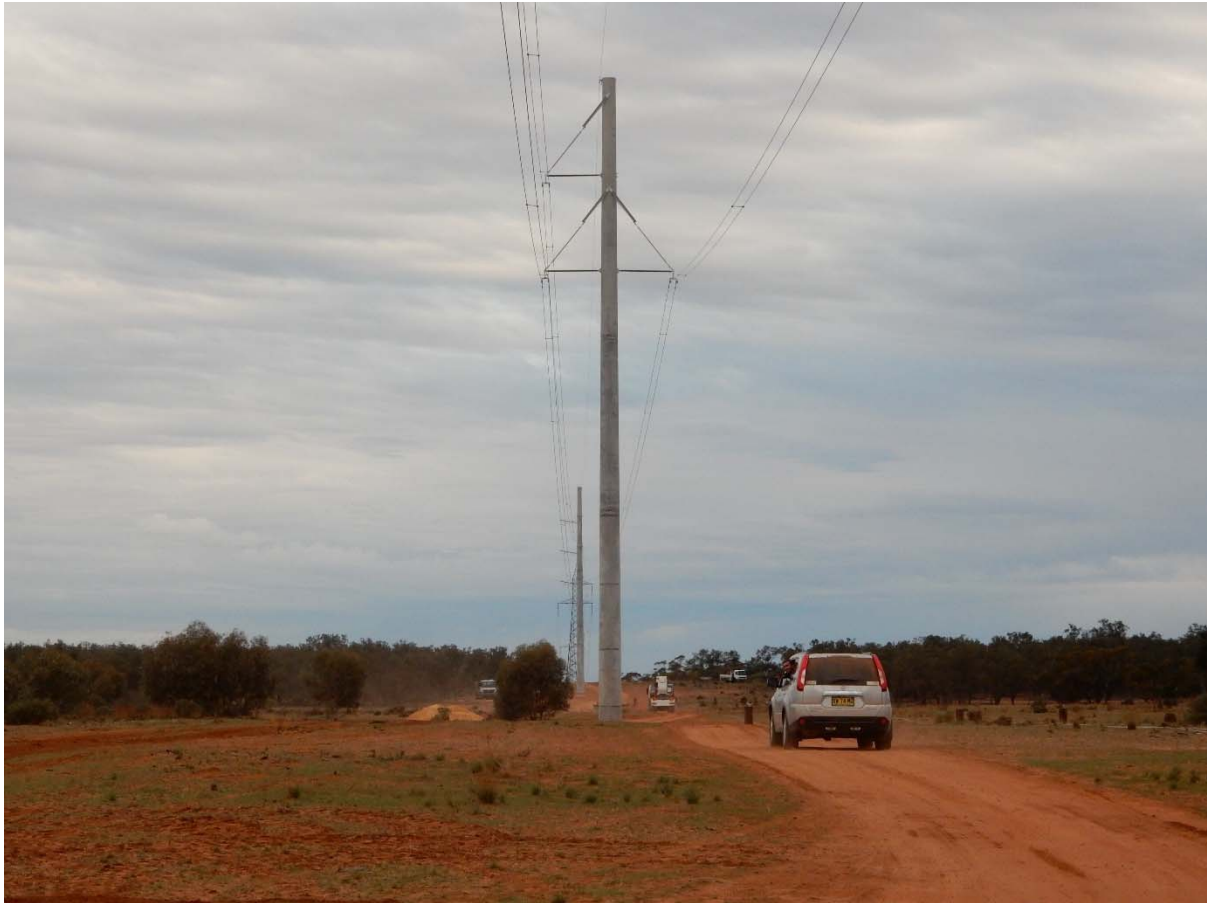
Figure 3-17 Example of overhead powerline
