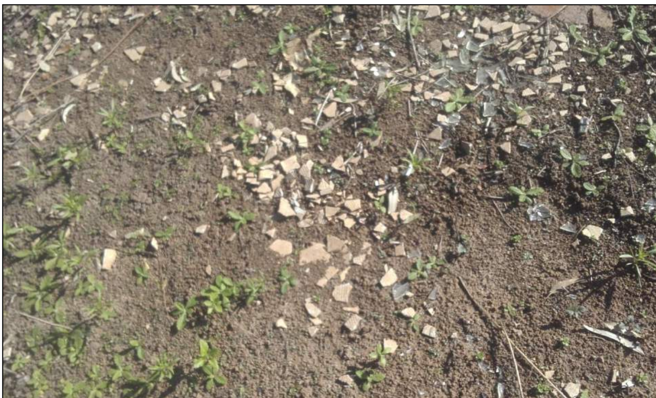
Photograph 4 – Western section of Lot 19/20, scattered, poor condition presumed asbestos debris on soil surface.
