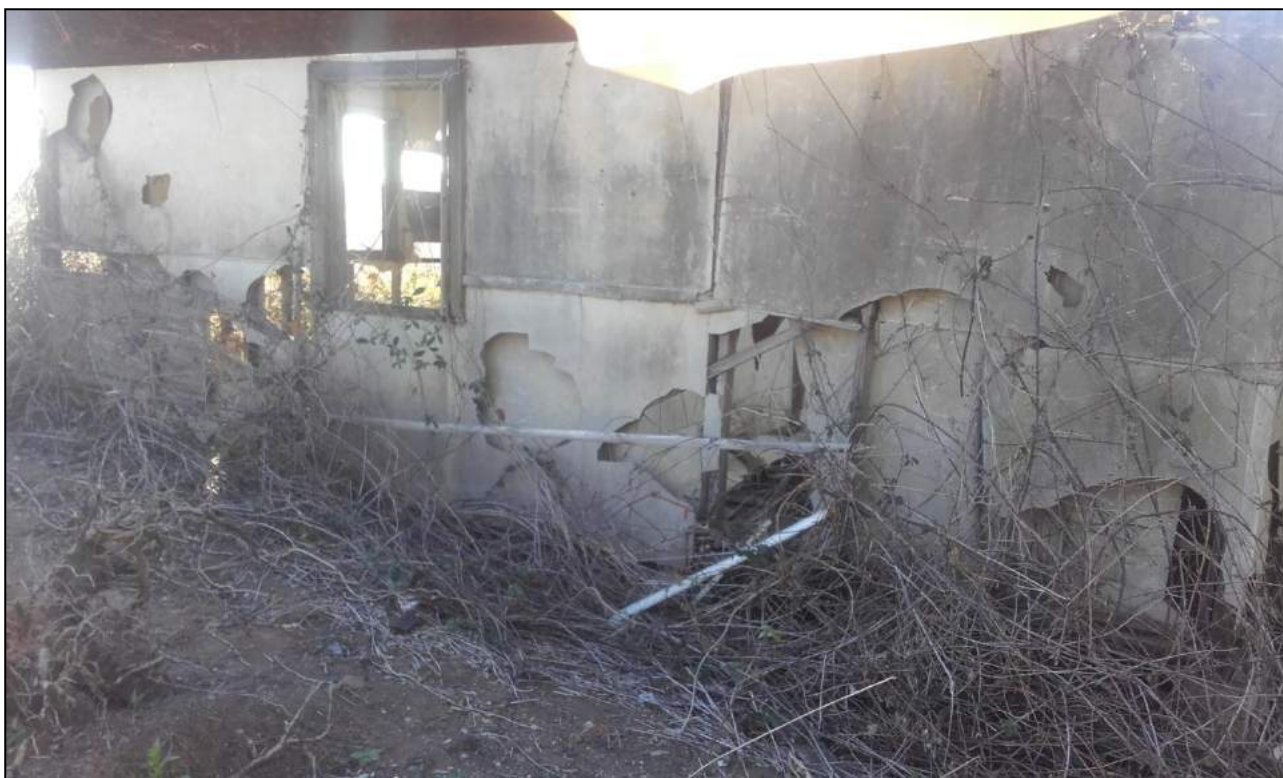
Photograph 1 – Northern section of Site (Lot 18), degraded fibro shed, with presumed poor condition asbestos debris on surrounding soil surface.
