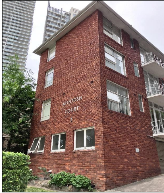
Photograph 15: 3 Help Street, exterior, eave linings generally, fibre cement sheeting, suspected asbestos.
