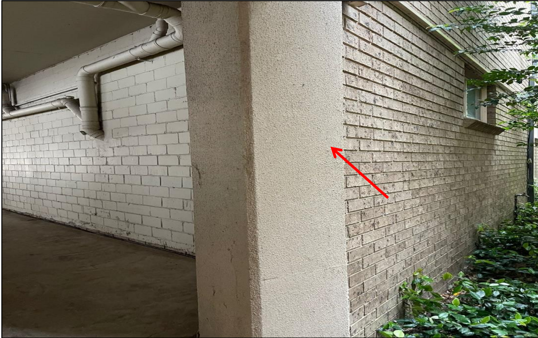
Photograph 13: 5 Help Street, exterior, car park area, column, textured coating, no asbestos detected by analysis.
