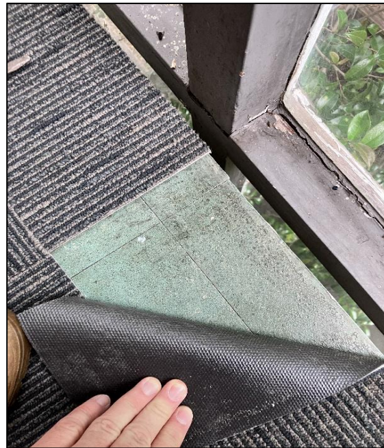
Photograph 4: 3 Help Street, stairwells generally, landings and stairs, floor, below carpet, vinyl tiles, suspected asbestos.
