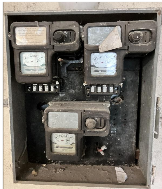
Photograph 10: 3 Help Street, interior, ground floor, Laundry, electrical panel, resinous board(s), suspected asbestos.
