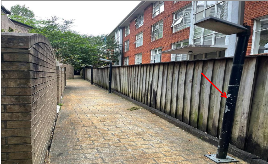
Photograph 23: 5 Help Street, exterior, eastern passageway, light post, black paint, lead paint detected by analysis.
