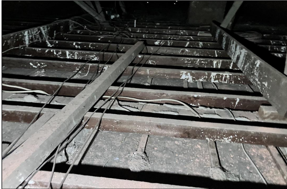
Photograph 21: 3 Help Street, roof cavity, top of ceiling, settled dust/debris, lead detected (130 mg/m 2 ).
