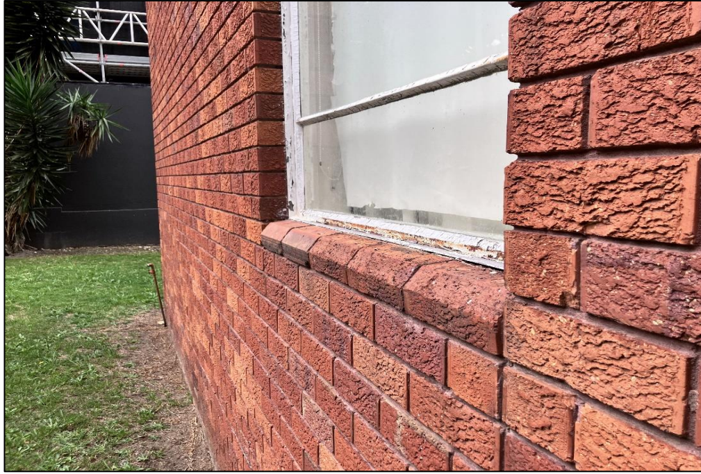
Photograph 1: 3 Help Street, exterior, northern façade, ground floor, window frame, glazing putty, no asbestos detected by analysis.
