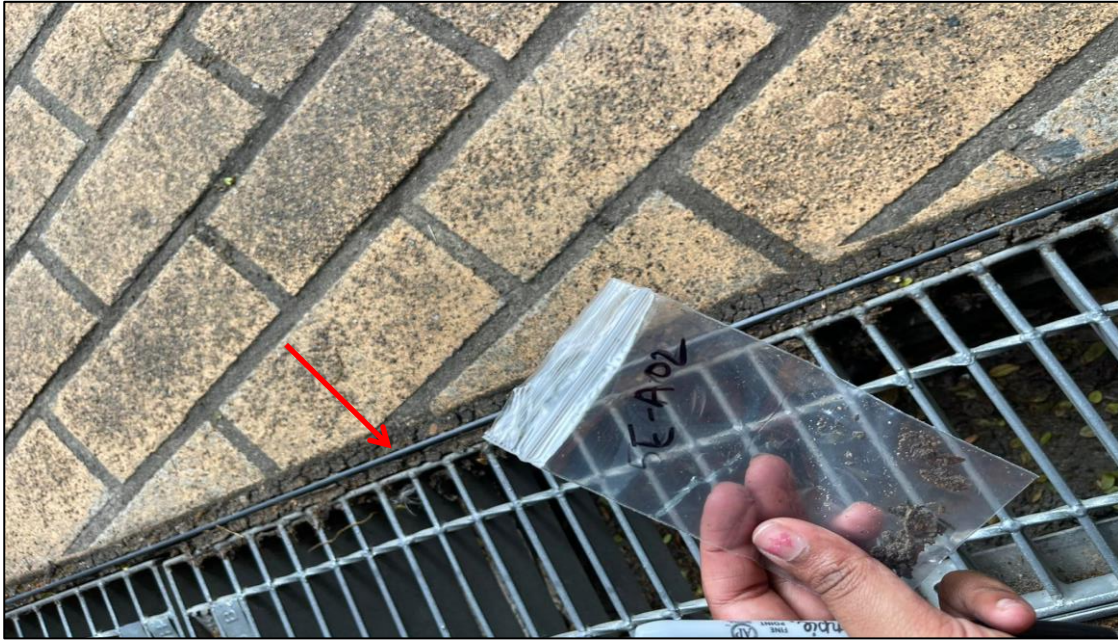
Photograph 11: 5 Help Street, exterior, stormwater drain lining, adhesive-like material, no asbestos detected by analysis.
