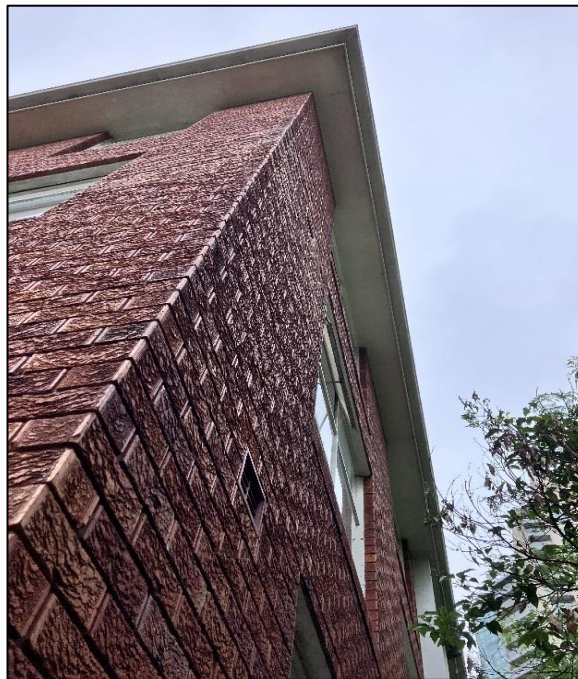
Photograph 14: 3 Help Street, exterior, eave linings generally, fibre cement sheeting, suspected asbestos.
