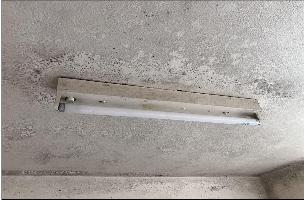
Photograph 23: 3 Help Street, ground floor, Laundry, fluorescent light fittings, internal components (e.g., capacitors), PCB (suspected).
