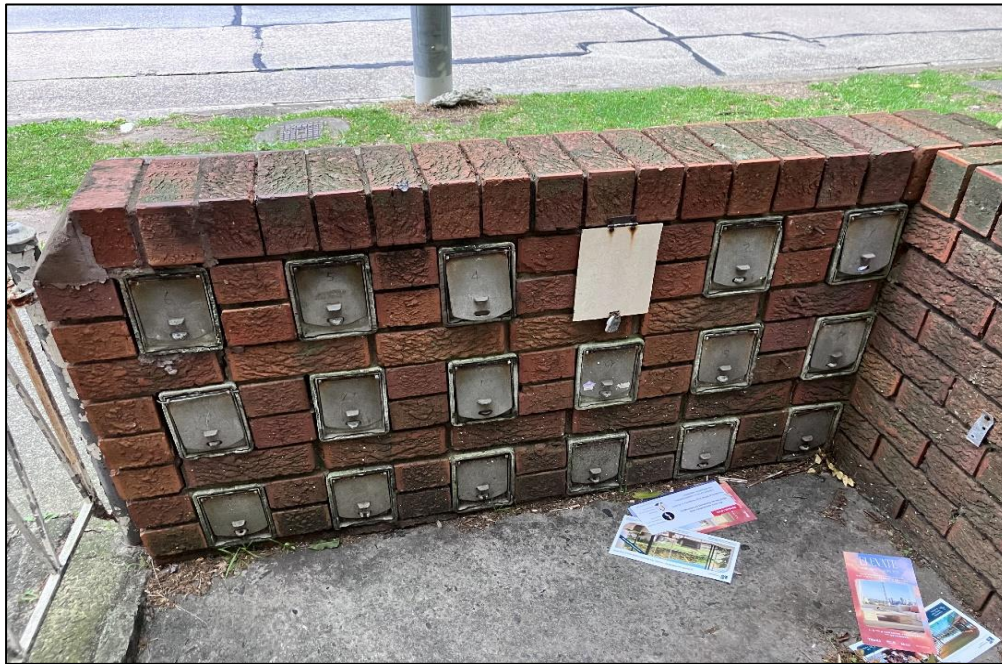
Photograph 12: 3 Help Street, exterior, southern yard, mailbox linings, fibre cement product, asbestos detected by analysis.
