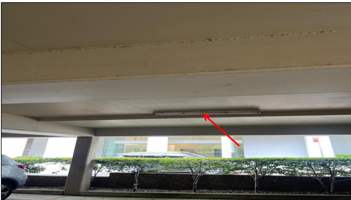
Photograph 18: 5 Help Street, exterior, car park area, ceiling, fluorescent light fittings, internal components (e.g., capacitors / ballasts), PCB (suspected).
