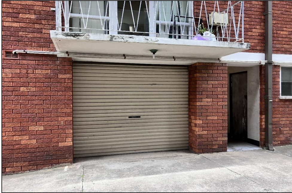
Photograph 25: 3 Help Street, ground floor, garages, suspected fluorescent light fittings, inaccessible (PCB suspected).
