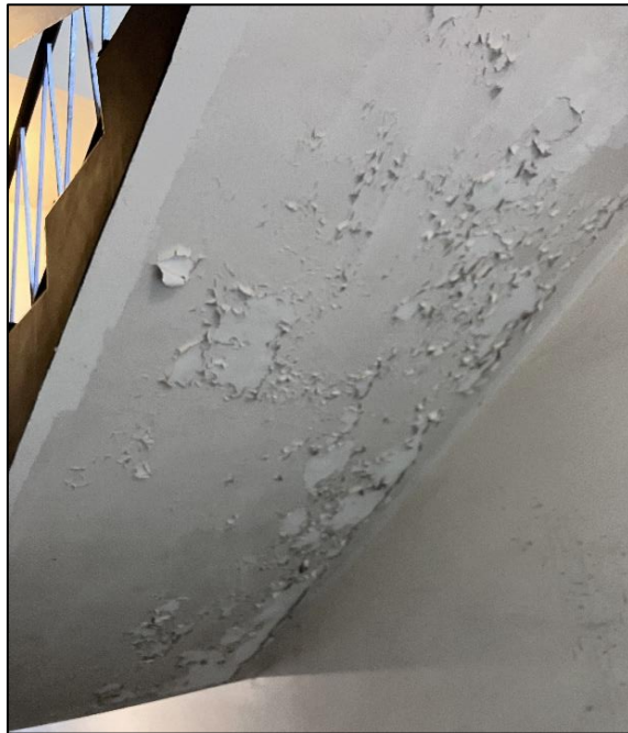
Photograph 20: 3 Help Street, interior, southern stairwell, ground floor, ceiling and base of stairwell, white paint, lead paint not detected.
