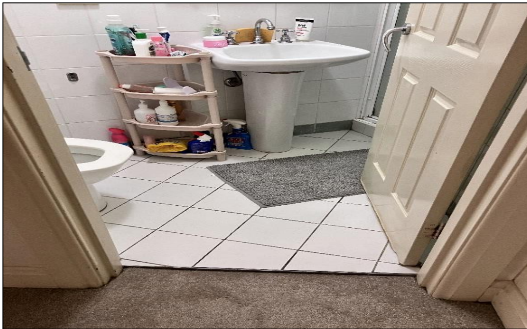
Photograph 2: 5 Help Street, Units 4, 11, 19 and 28, below ceramic tiled surfaces (e.g. walls, floors, bath surrounds), substrate, inaccessible.
