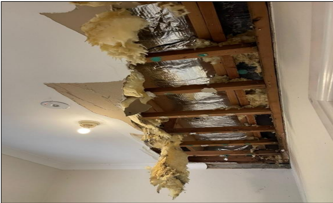
Photograph 17: 5 Help Street, Level 1, southern stairway, ceiling cavity insulation, no asbestos detected by analysis (SMF detected).
