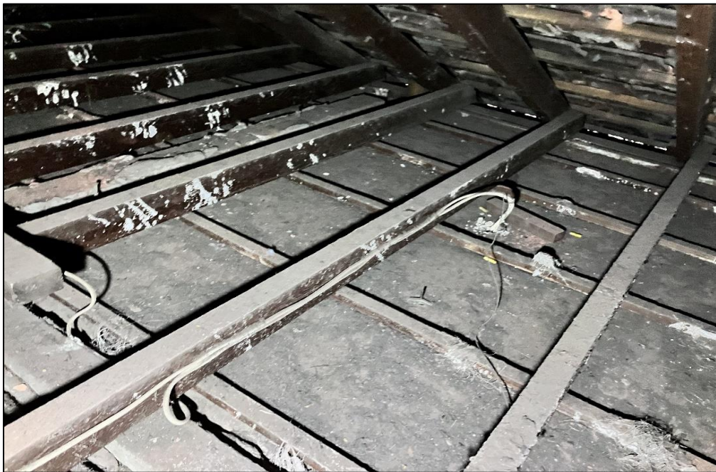
Photograph 22: 3 Help Street, roof cavity, top of ceiling, settled dust/debris, lead detected (130 mg/m 2 ).
