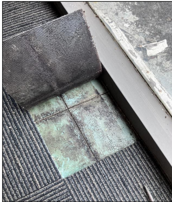
Photograph 2: 3 Help Street, stairwells generally, landings and stairs, floor, below carpet, vinyl tiles, suspected asbestos.
