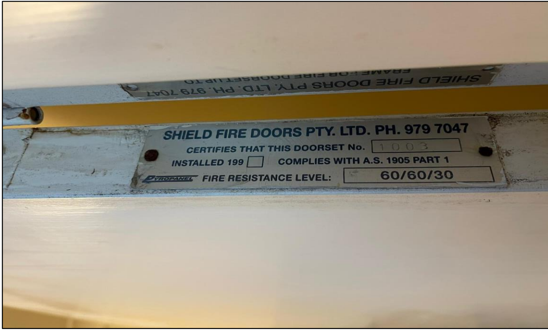
Photograph 21: 5 Help Street, generally, fire door (s), insulation, suspected asbestos.
