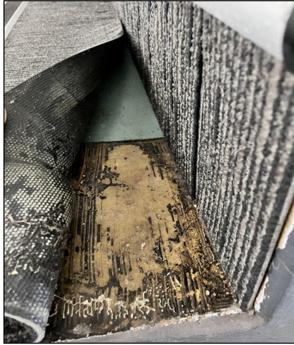
Photograph 3: 3 Help Street, stairwells generally, landings and stairs, floor, below carpet, vinyl tiles, suspected asbestos.
