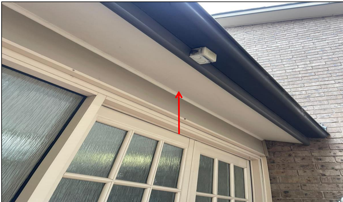
Photograph 16: 5 Help Street, exterior, level 1 staircase, eaves, fibre cement sheeting, no asbestos detected by analysis.
