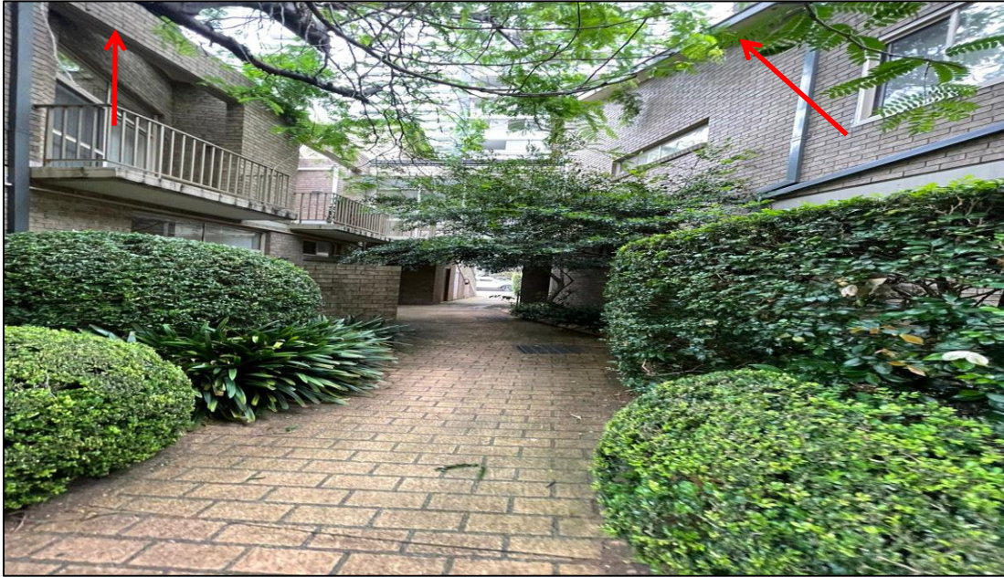
Photograph 9: 5 Help Street, exterior, eave linings generally, fibre cement sheeting, inaccessible suspected asbestos
