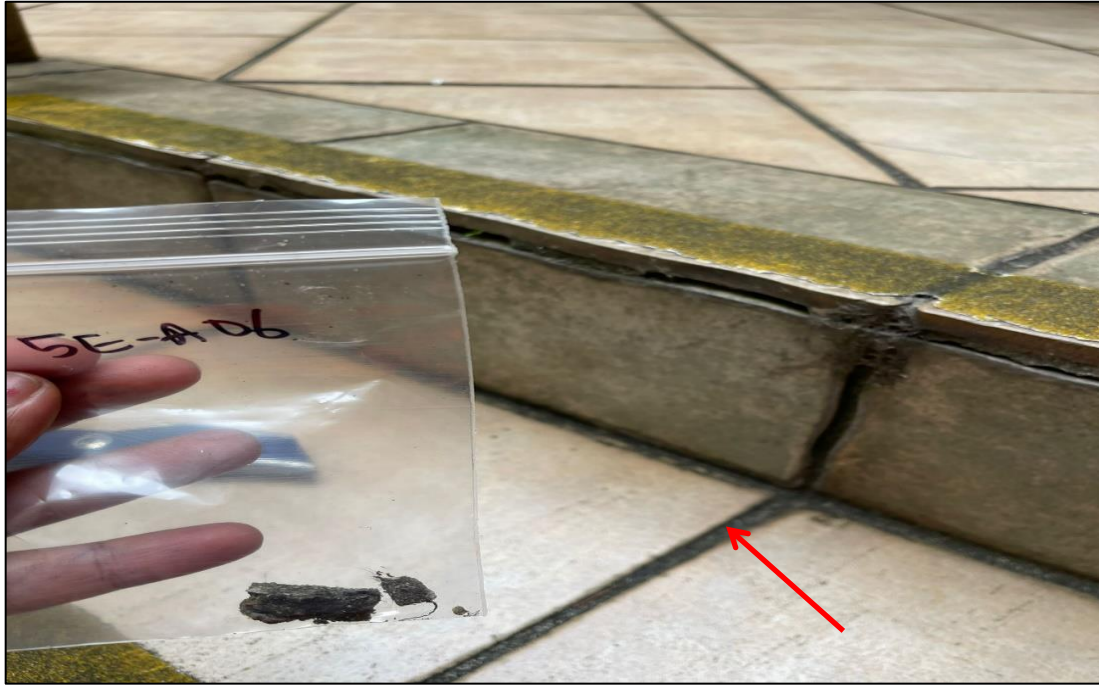
Photograph 15: 5 Help Street, exterior, level 1 staircase, stairs, joint, cement material, no asbestos detected by analysis.
