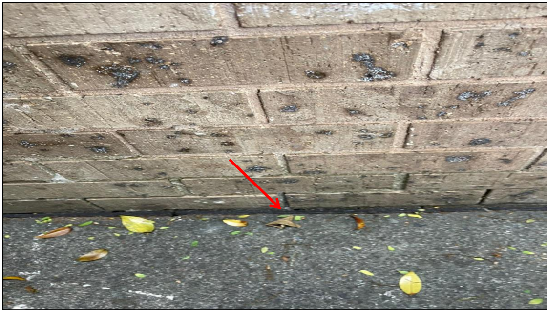
Photograph 10: 5 Help Street, exterior, joining between floor and wall, black bituminous material, no asbestos detected by analysis.
