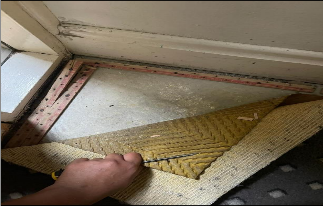
Photograph 19: 5 Help Street, stairwells / flooring generally, landings and stairs), floor, below carpet, concrete flooring, suspected non-asbestos.
