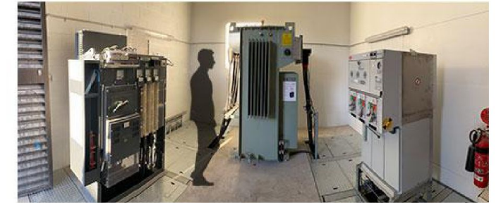
Inside a chamber substation
