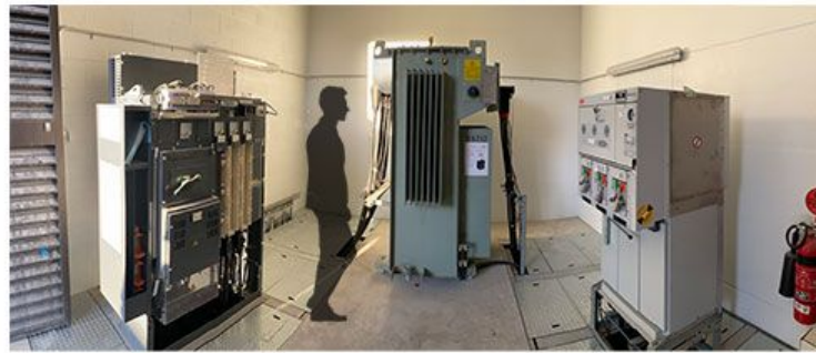
Inside a chamber substation
