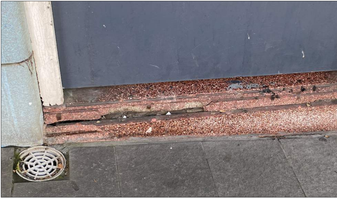
Fig. 11. Damaged door threshold in Atchison Street.
