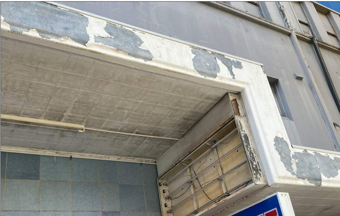
Fig. 38. Awning fascia is to be repaired prior to proper preparation and repainting. Redundant signage is to be removed or reinstated.
