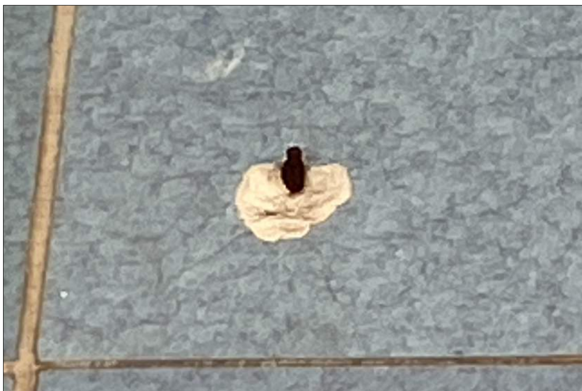
Fig. 6. Broken tiles are to be replaced with matching tiles or repaired if no suitable tile is available. Rusting fixing are to be removed from the tiles and the holes repaired.
