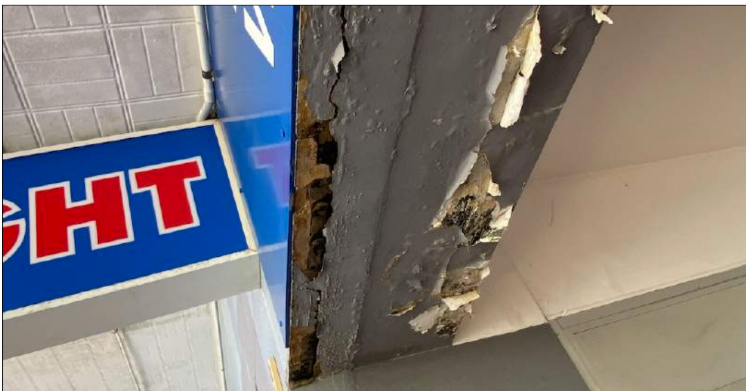
Fig. 10. Awning water penetration of the concrete beam over the Atchison Street entry.
