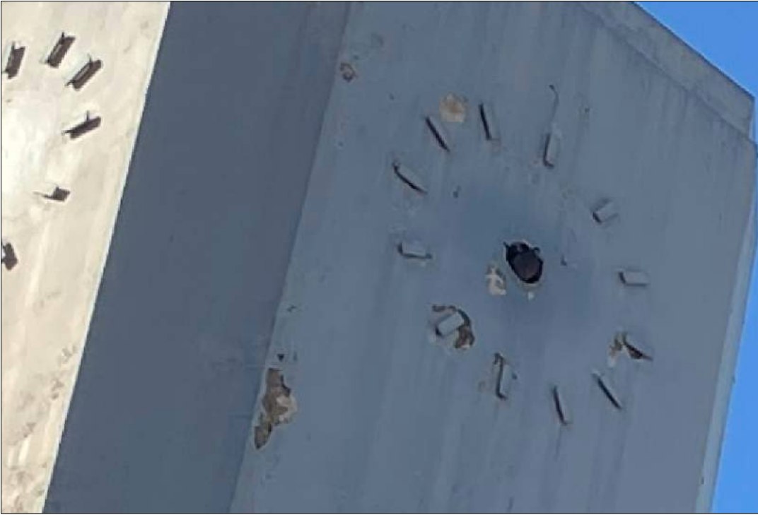
Fig. 33. The pigeons are to be removed from inside the clock tower and damaged concrete is to be repaired.
