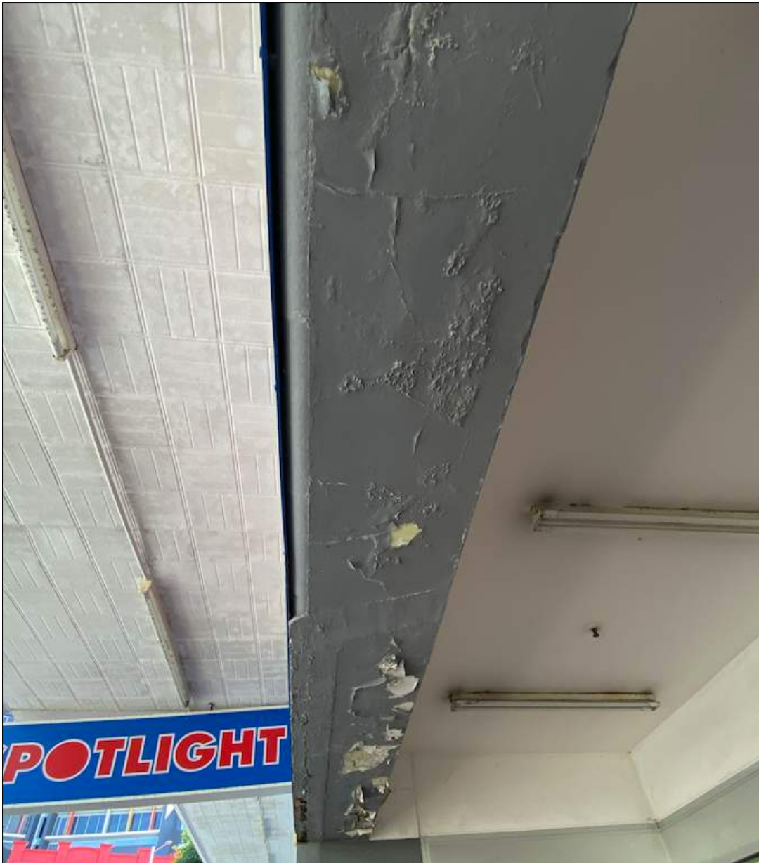
Fig. 9. Awning water penetration of the concrete beam over the Atchison Street entry.
