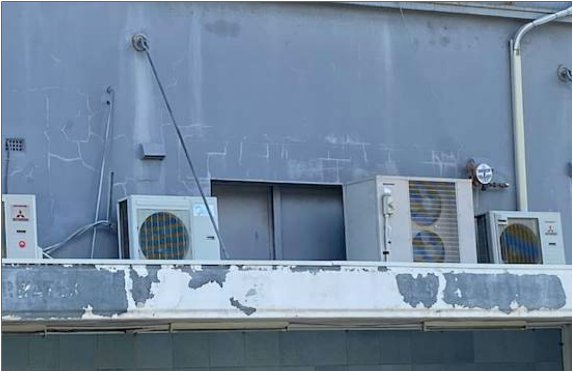
Fig. 23. Cracked, crazed and damaged rendered masonry is to be repaired.
