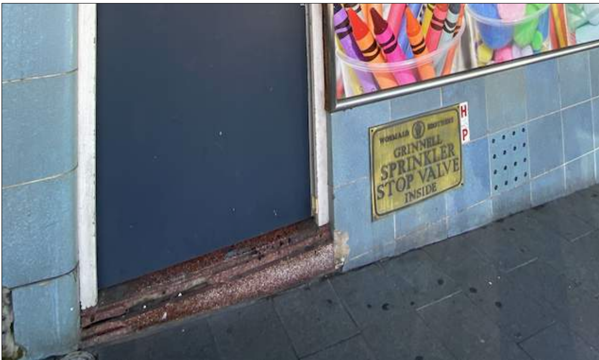
Fig. 12. Damaged door threshold in Atchison Street.
