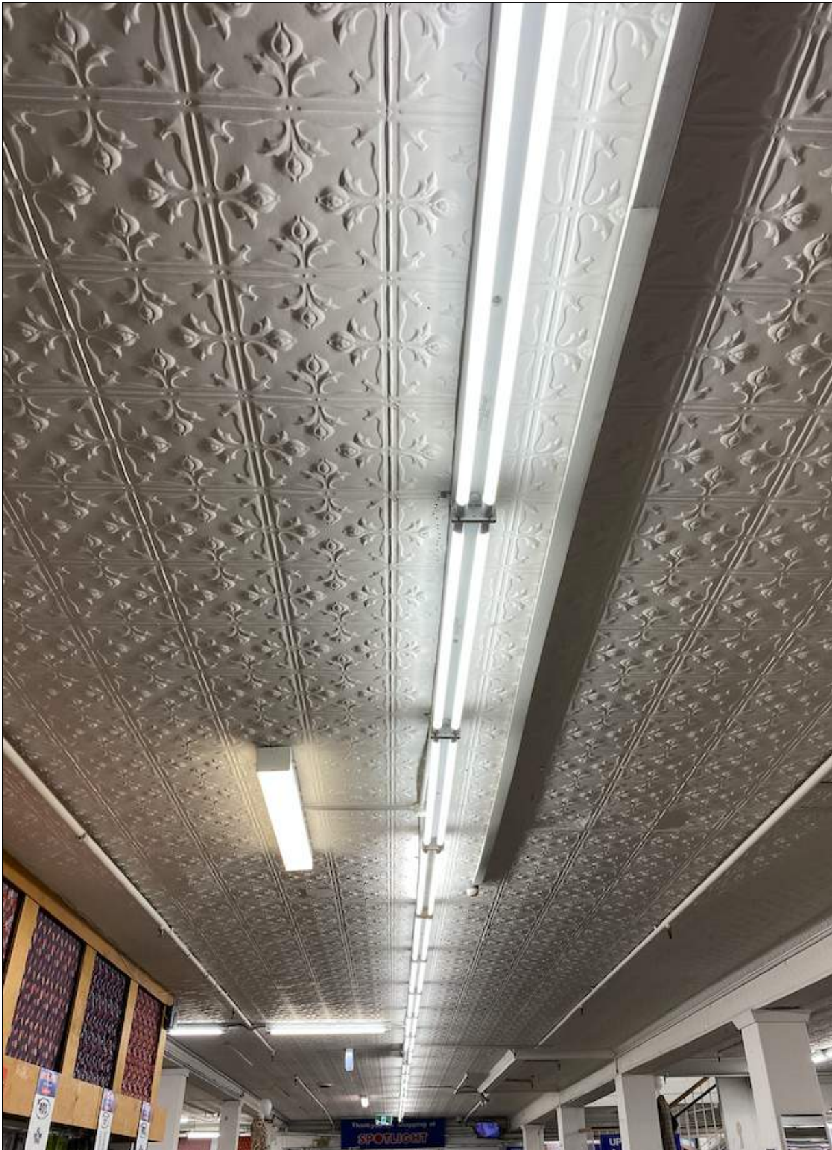
Fig. 44. The pressed metal ceilings of the lower ground floor are to be salvaged where ever possible, protected from damaged and recycled either in the new construction in a nominated area or delivered to a heritage building centre.
