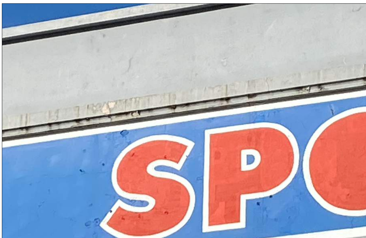
Fig. 20. All rusting remnants of redundant masonry anchors are to be removed from the facade on both Atchison and Crown Street.
