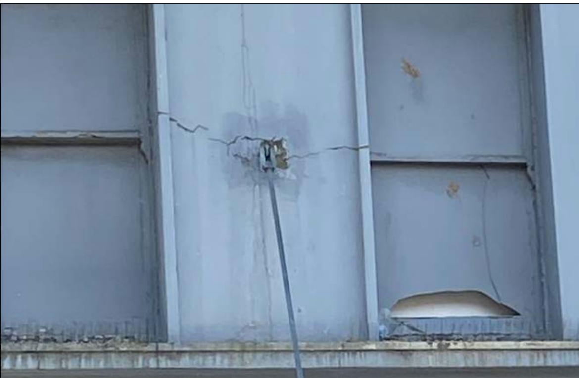
Fig. 22. Cracked, crazed and damaged rendered masonry is to be repaired.
