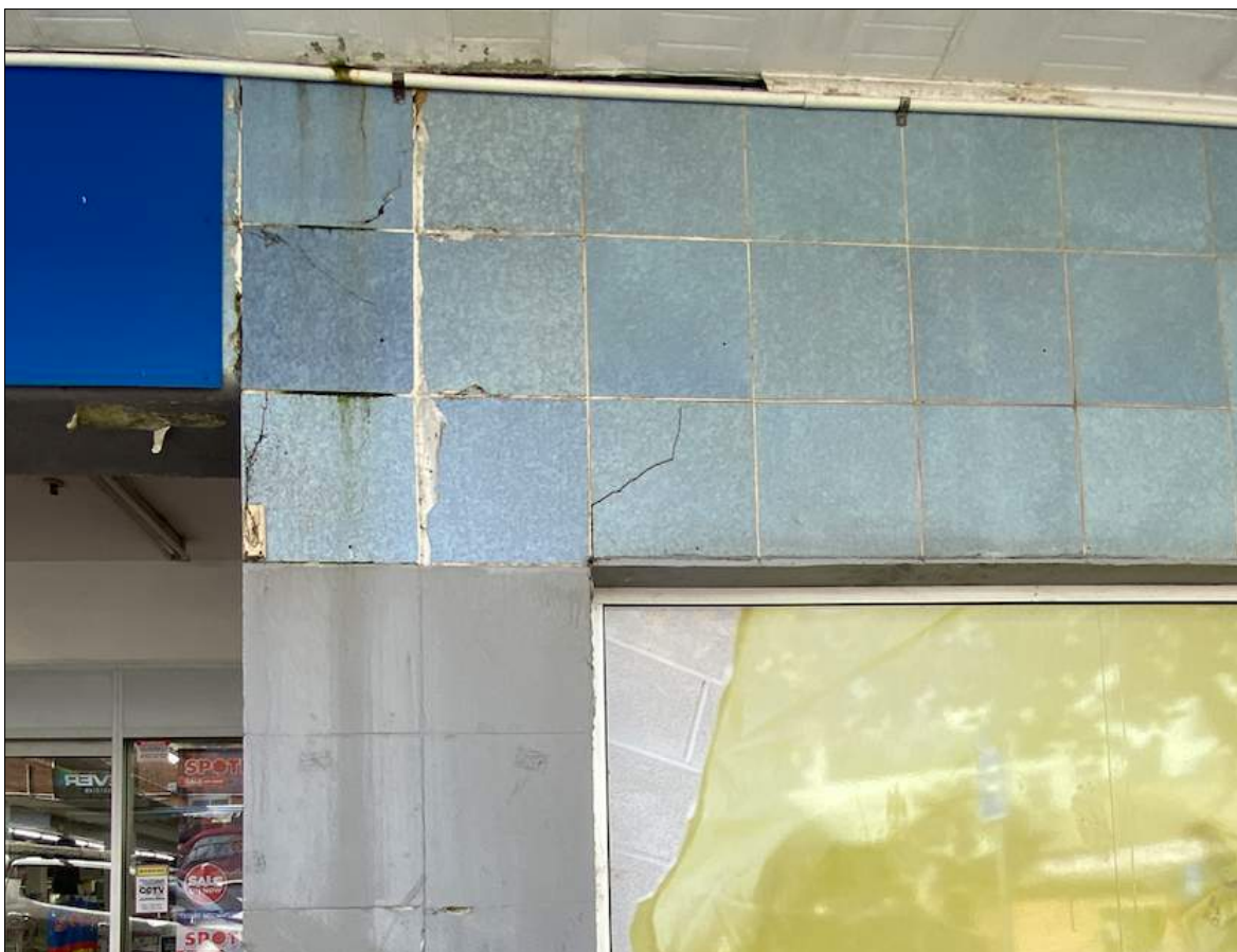
Fig. 7. Broken tiles are to be replaced with matching tiles or repaired if no suitable tile is available. Surface conduits are to be removed from façade and the damage made good.
