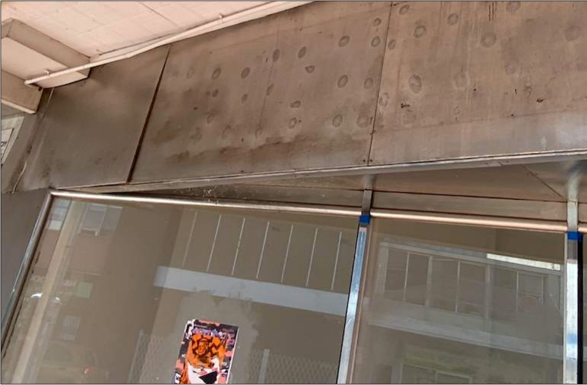
Fig. 15. Sections of the stainless steel cladding above the shopfront glazing are to be removed to reveal the underlying surface, Guidance from the nominated heritage consultant is to be sort on how these areas are to be treated.
