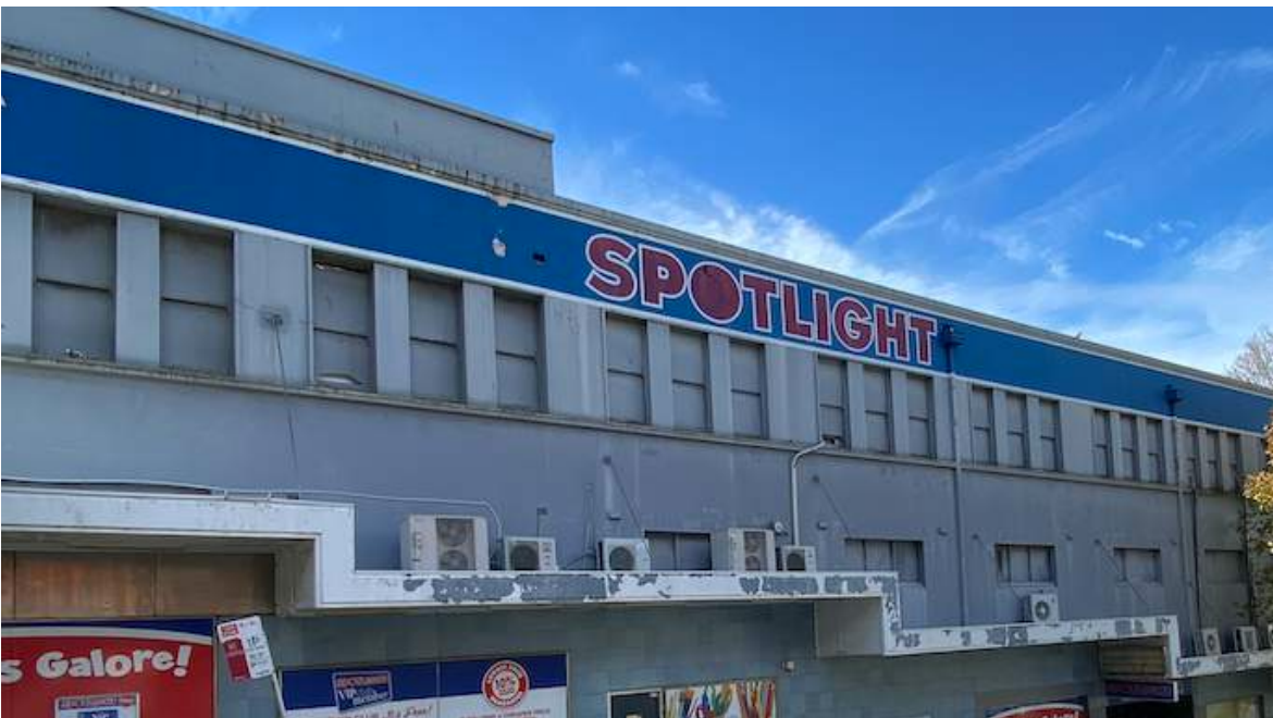
Fig. 18. All air-conditioning compressors, conduits, air-conditioning pipework, redundant brackets and fixings are to be removed from the facade on both Atchison and Crown Street.
