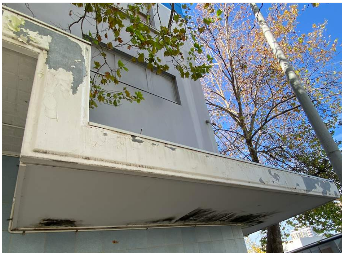
Fig. 35. Evidence on numerous areas on the underside of the shop awning suggests that the awning roof and guttering has rusted out and needs to be replaced.
