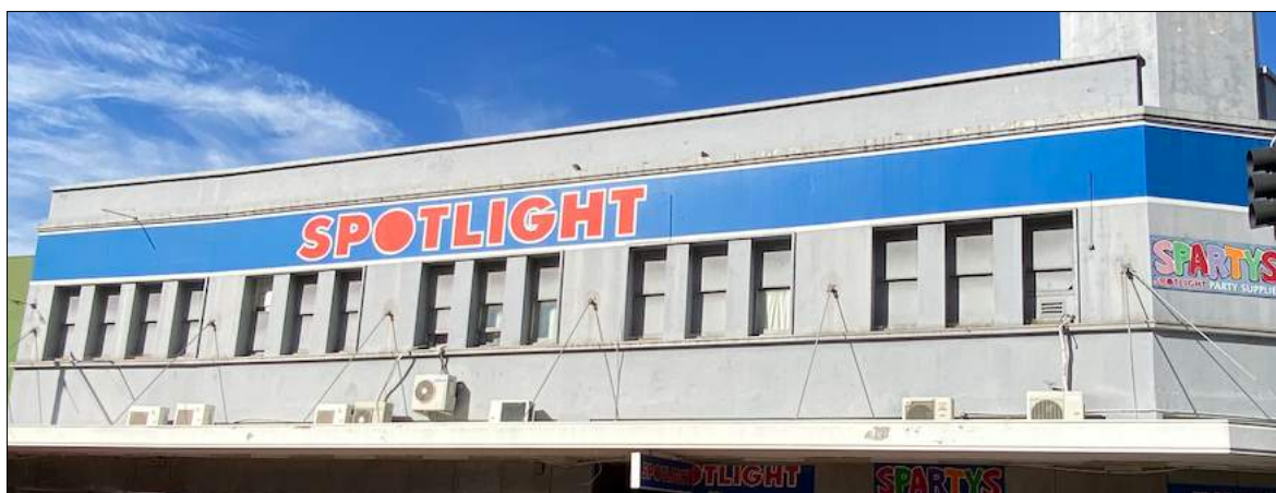
Fig. 19. All air-conditioning compressors, conduits, air-conditioning pipework, redundant brackets and fixings are to be removed from the facade on both Atchison and Crown Street.
