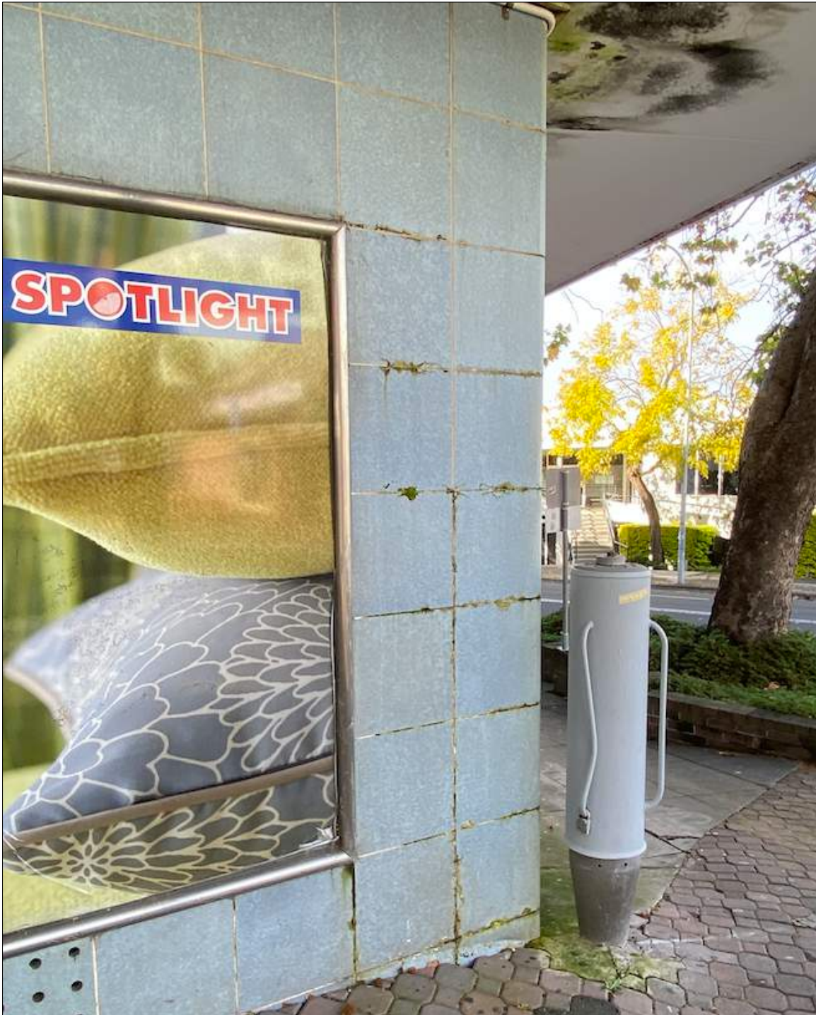
Fig. 4. The façade wall tiling is to be cleaned. The curved stainless steel shopfront glazing trim is to be retained and protected from damage for the duration of any and all approved building works.
