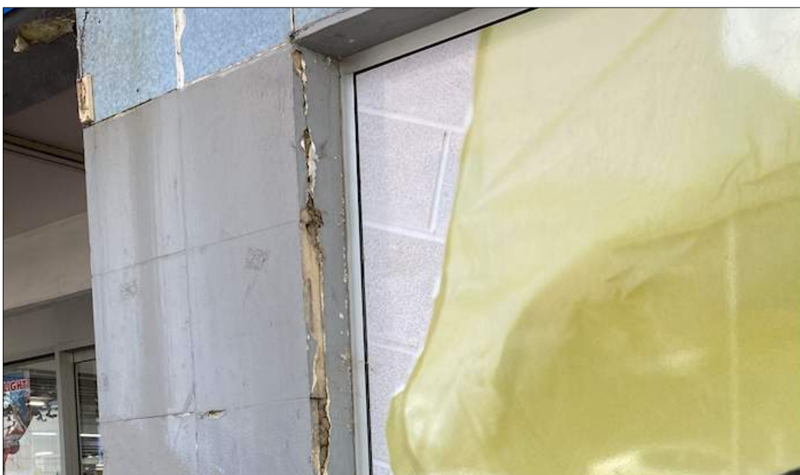
Fig. 8. Damaged painted render to shop fronts in Atchison Street.
