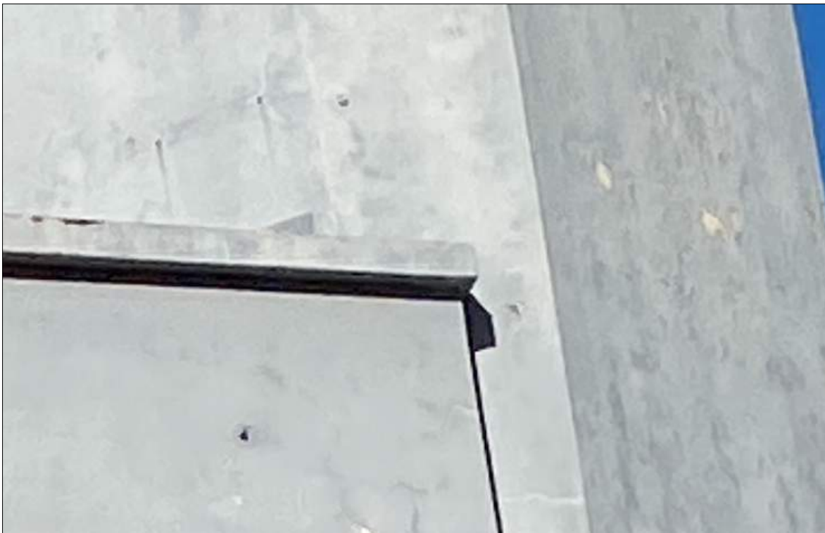
Fig. 32. All rusting remnants of redundant masonry anchors are to be removed from the clock tower.
