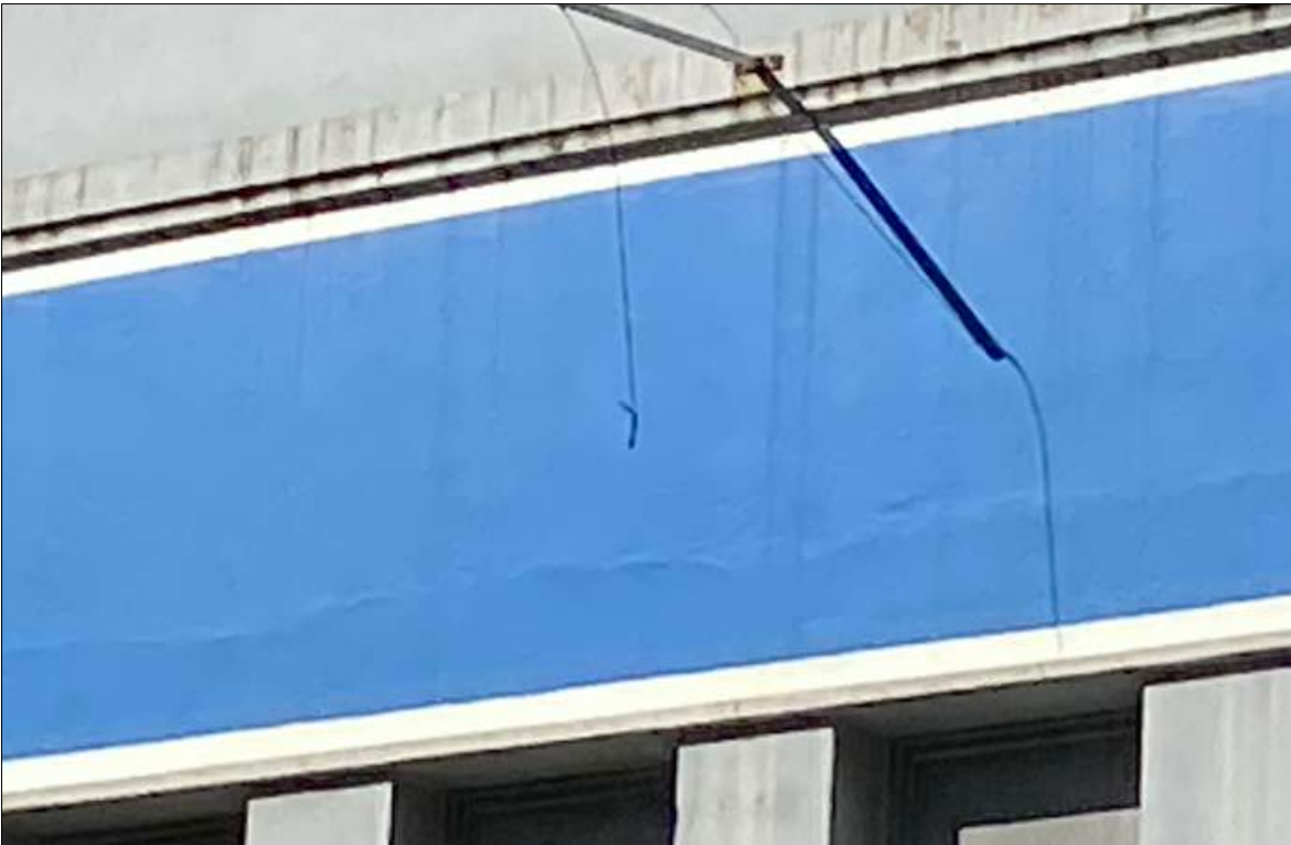
Fig. 21. The deformity in the painted render on eastern end on the Crown Street façade is to be investigated and findings reported to the nominated heritage consultant and guidance sort on any required remediation.
