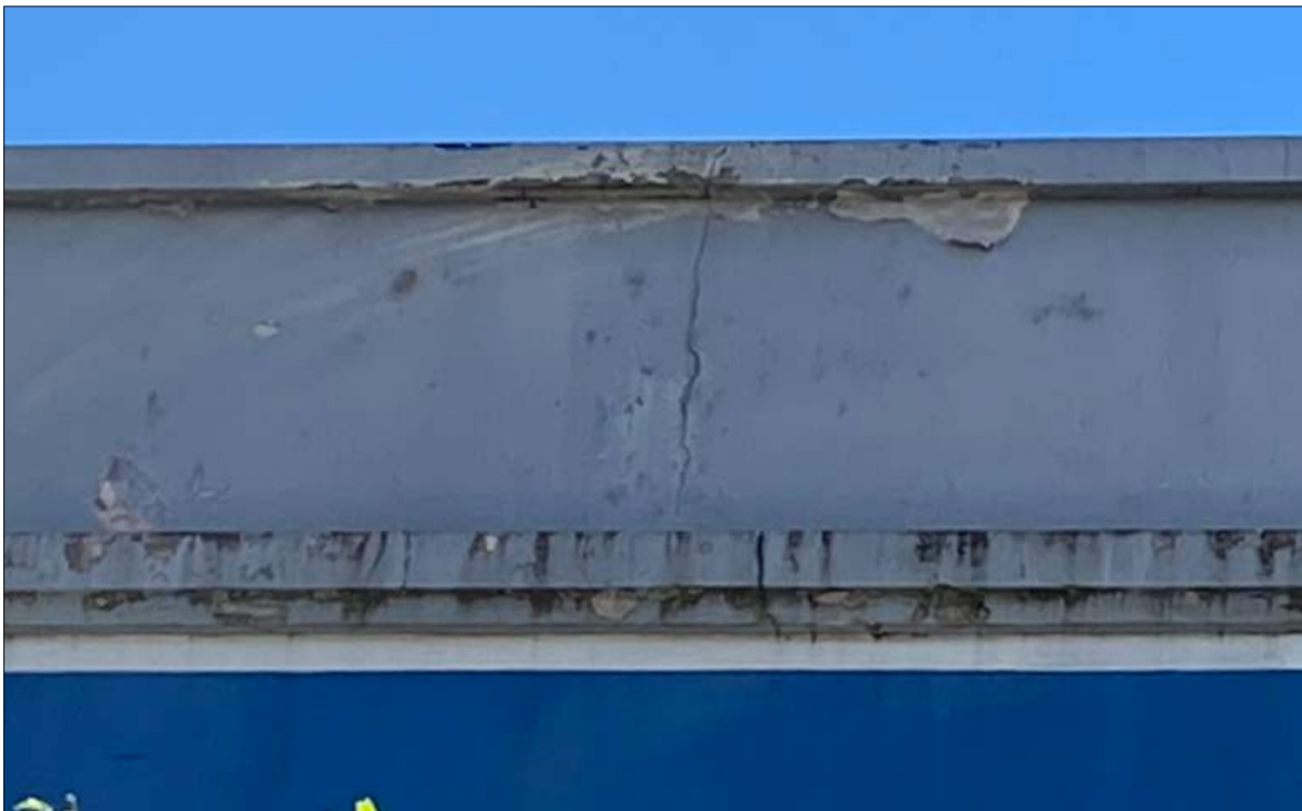
Fig. 24. Cracked, crazed and damaged rendered masonry is to be repaired.
