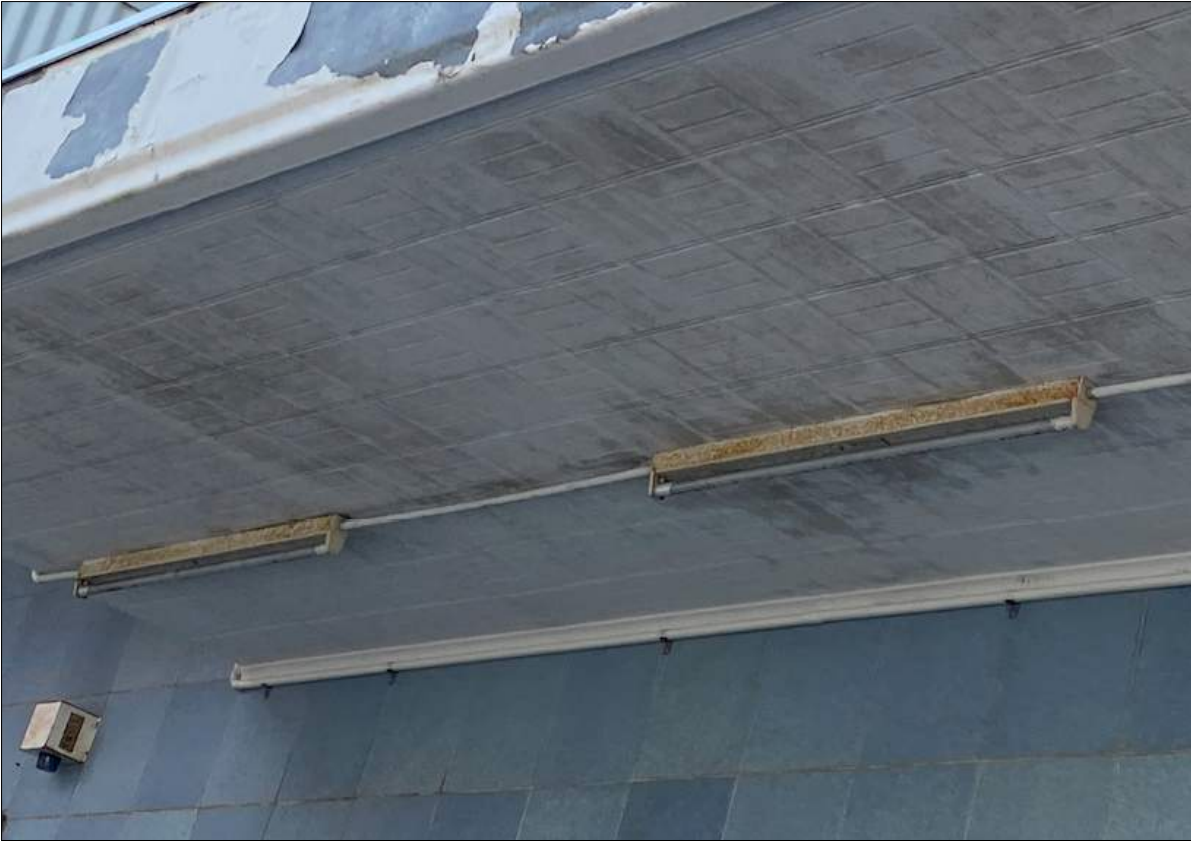
Fig. 42. Rusting and damaged awning soffits lighting is to be replaced. Guidance from the nominated heritage consultant is to be sort on what replacement lighting is appropriate.
