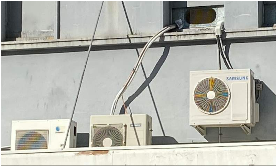
Fig. 17. All air-conditioning compressors, conduits, air-conditioning pipework, redundant brackets and fixings are to be removed from the facade on both Atchison and Crown Street.
