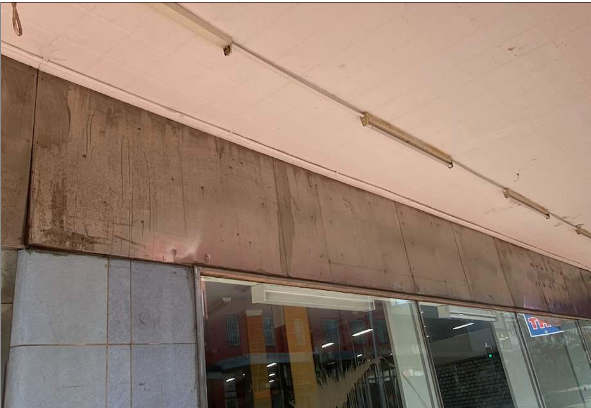
Fig. 16. Sections of the stainless steel cladding above the shopfront glazing are to be removed to reveal the underlying surface, Guidance from the nominated heritage consultant is to be sort on how these areas are to be treated.
