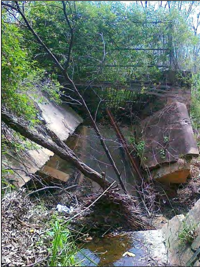
Plate 2-3: Channel Failure and Scouring Upstream (Eastward)
