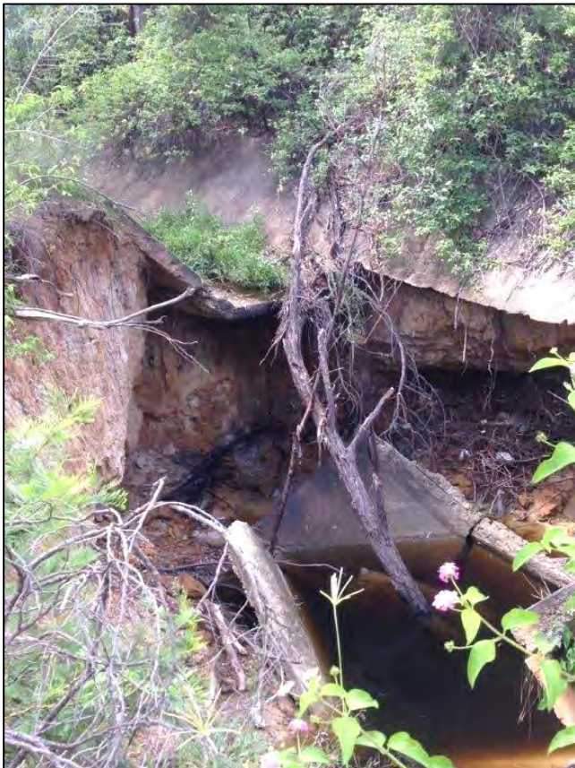
Plate 2-4: Channel Failure and Scouring Viewing Downstream (Westward)
