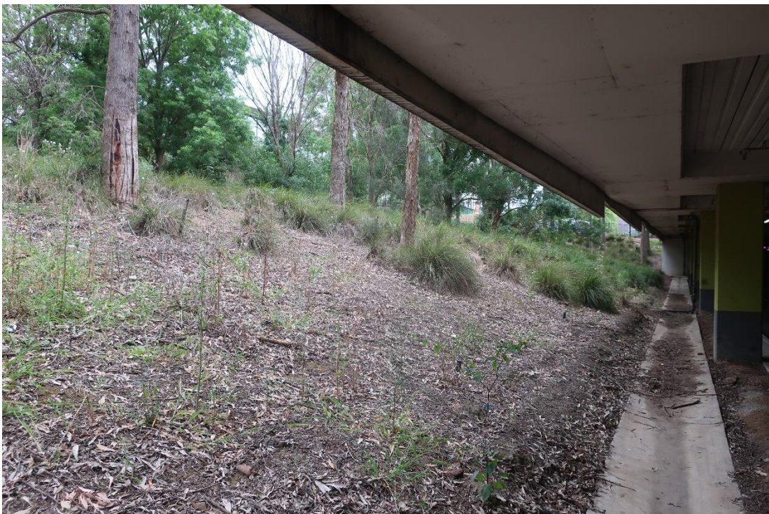
Figure 1.13 Northern boundary of study area, showing current open slop down to town centre basement level car park. Facing west. AMAC Group, 14/10/2024, digital image 8780.
