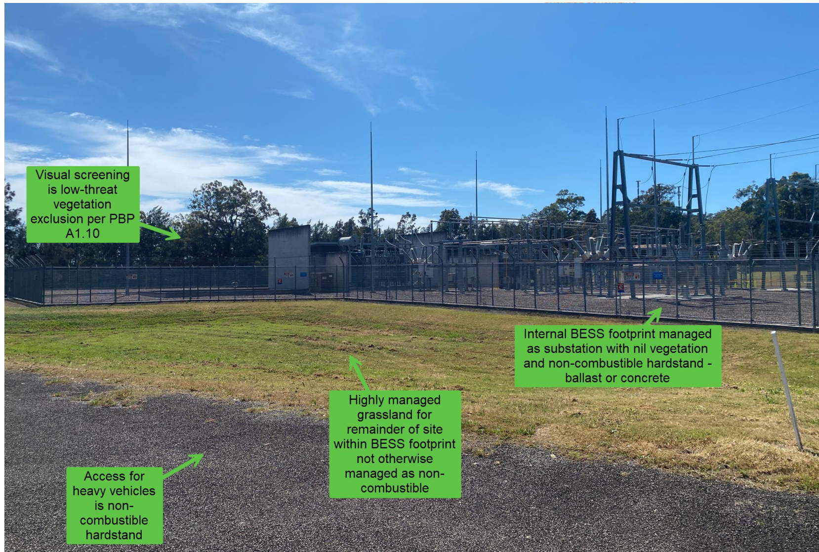
Figure 18: Landscaping management at typical Zone Substation demonstrating BESS footprint treatment
