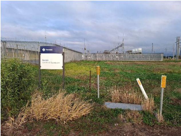
Plate 6.5 Substation on the southern side of Stoney Creek Road, view south
