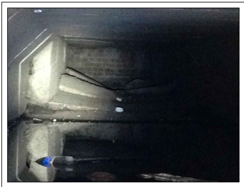
OBSTRUCTION INSIDE 1800 CULVERT
