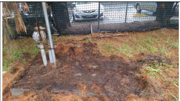
Photo 2: concrete slab with hand pump and vent pipe.
