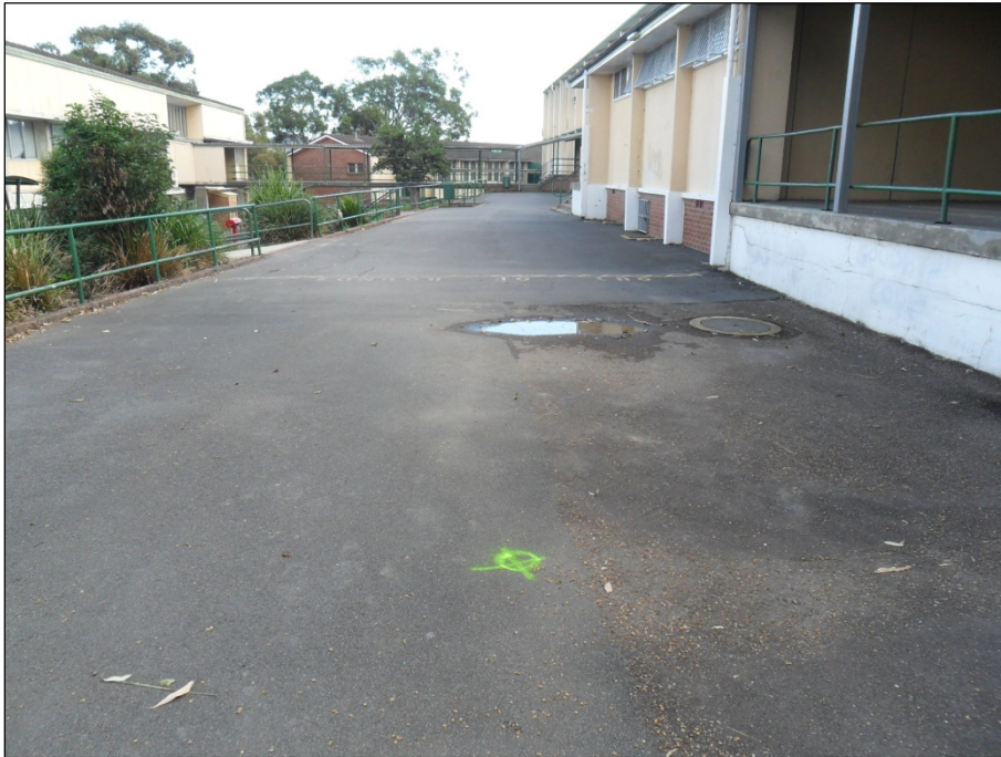
Figure 5: Paved area in the central-northern portion of the site (former demolition area)
