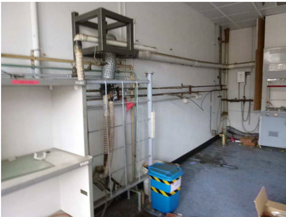
Plate 6: Metal pipes on the walls of some of the laboratories within Materials Science Building (E8) for compressed gases and cooling water delivery.
