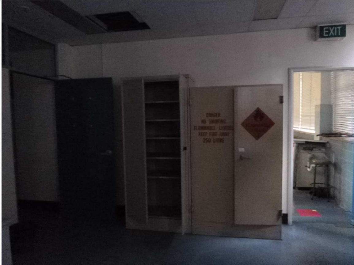
Plate 3: Cabinet which had stored chemicals within a laboratory within the Materials Science Building (E8). Similar cabinets are located in some of the various laboratories located within the building.
