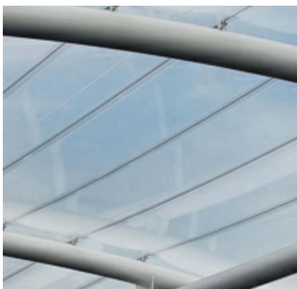
RES AQUATICS HALL ROOF ETFE ROOFING SYSTEM
