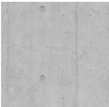
COF MULTIPLE LOCATIONS CONCRETE OFF-FORM
