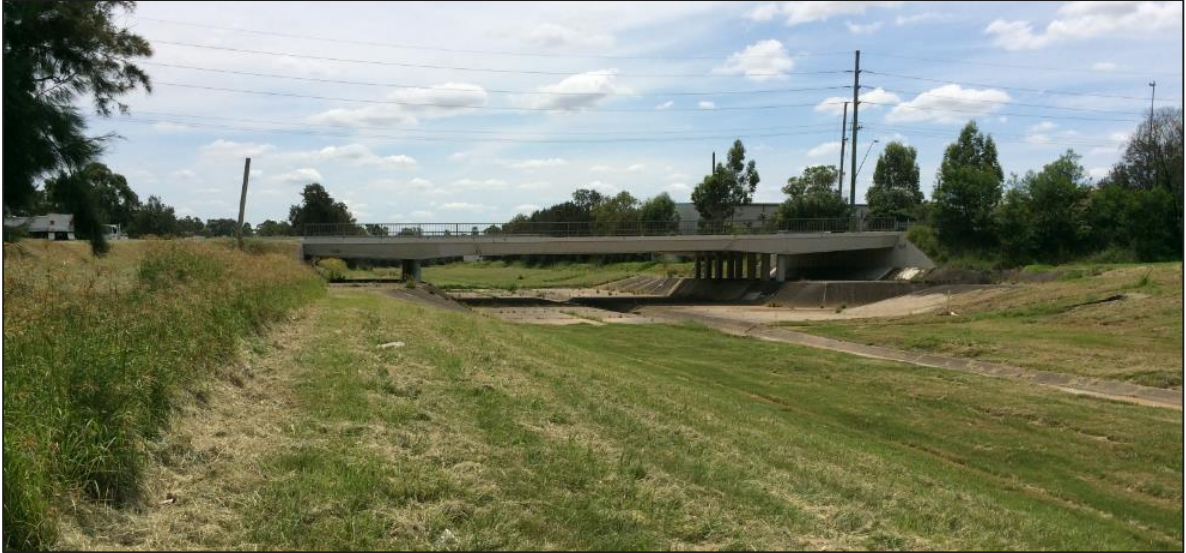
Photo 2: Bow Bowing Creek, Airds Road bridge viewing northward (downstream) along the western site boundary.
