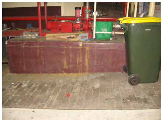
Figure 3.69 Fire services equipment in the cart dock/loading dock near the Gresham Street entrance
