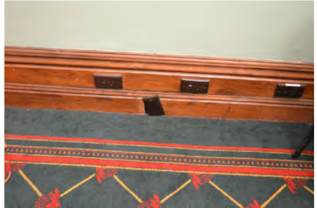
Figure 3.89 Typical socket outlets
