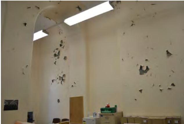
Figure 3.85 Example of failing paint in ground floor offices
