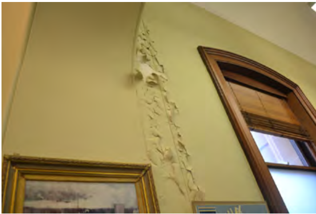
Figure 3.86 Example of failing paint in Bridge Street ground floor offices
