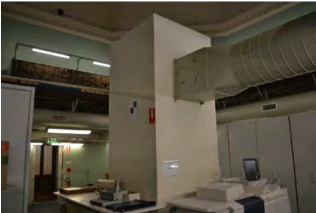
Figure 3.88 Service units in the central strong room
