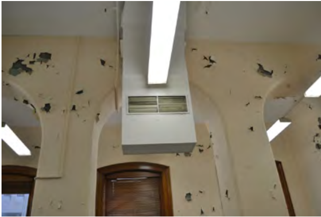
Figure 3.87 Air conditioning system in ground floor offices
