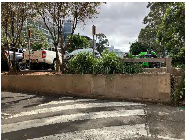
Figure 15 – View west showing the ground level vs car park level, indicating presence of fill to create carpark space
