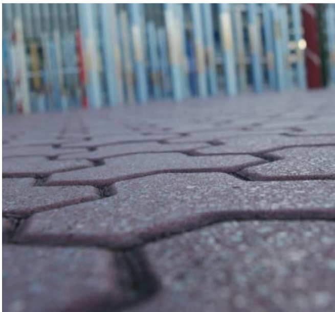
Trihex interlocking unit paving to match existing. Installed in accordance with SOP UEDM Section 3.1 Pavements.
