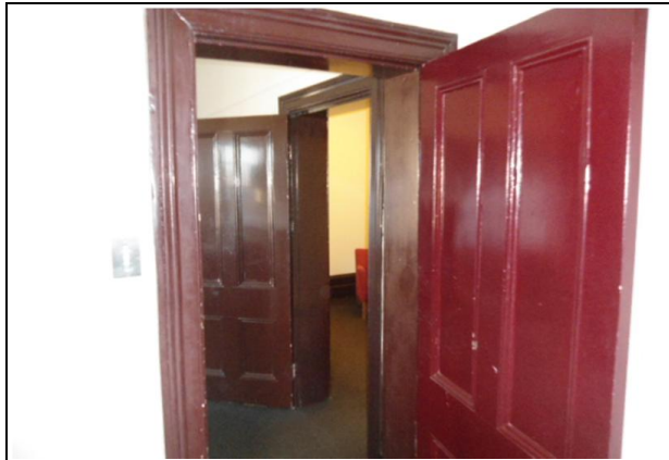
Photo No: J105234-H02-7912 Result: Lead Paint Presumed Positive
