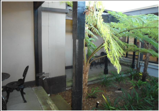
Photo No: J105234-H02-7924 Result: Lead Paint Positive
