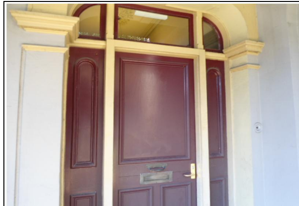
Photo No: J105234-H02-7928 Result: Lead Paint Presumed Positive
