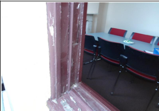
Photo No: J105234-H02-7916 Result: Lead Paint Positive 2.3%
