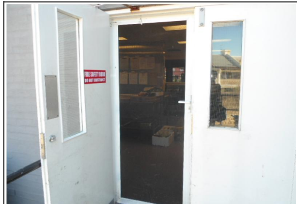
Photo No: J105234-H02-7925 Result: Asbestos Presumed Positive
