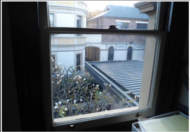
Photo No: J105234-H02-7909 Result: Lead Paint Positive 9.9%
