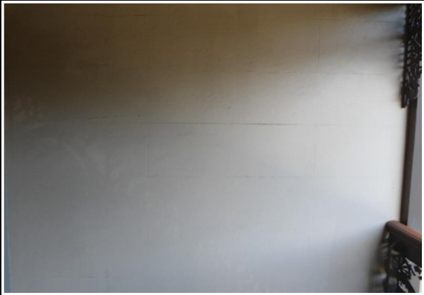
Photo No: J105234-H02-7919 Result: Lead Paint Positive
