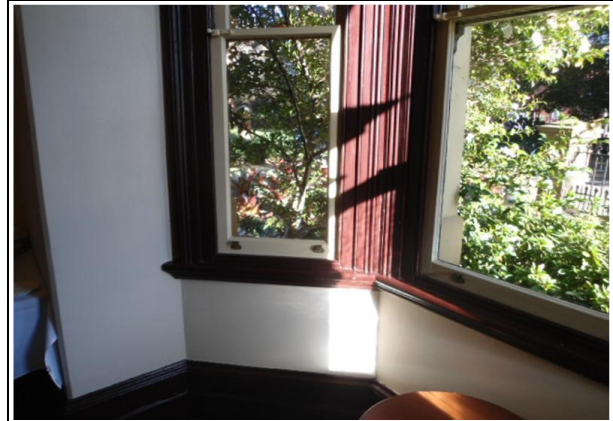
Photo No: J105234-H02-7921 Result: Lead Paint Presumed Positive
