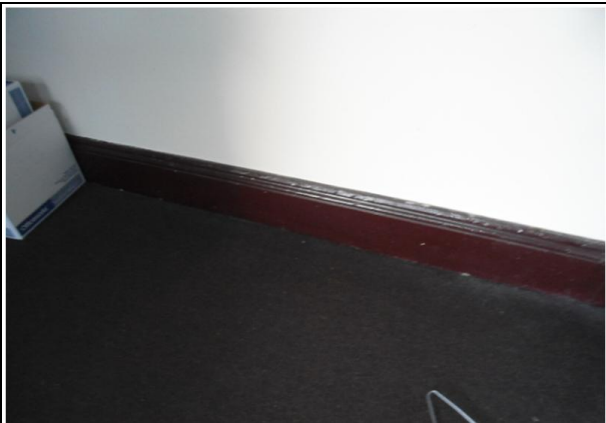
Photo No: J105234-H02-7911 Result: Lead Paint Presumed Positive
