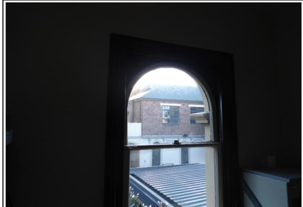
Photo No: J105234-H02-7910 Result: Lead Paint Positive 5.4%
