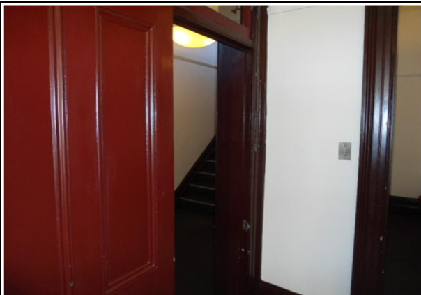
Photo No: J105234-H02-7922 Result: Lead Paint Presumed Positive
