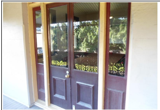
Photo No: J105234-H02-7917 Result: Lead Paint Presumed Positive
