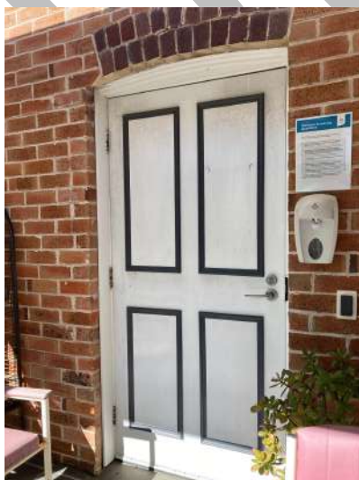
Figure 14: Photo of existing former Church contemporary door to be removed and infilled with like brickwork, recessed slightly back from the door opening. WPH.
