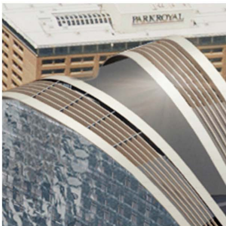
FT-5 Curved and faceted sun-shading profiles in aluminium LOCATION: East and West elevation
