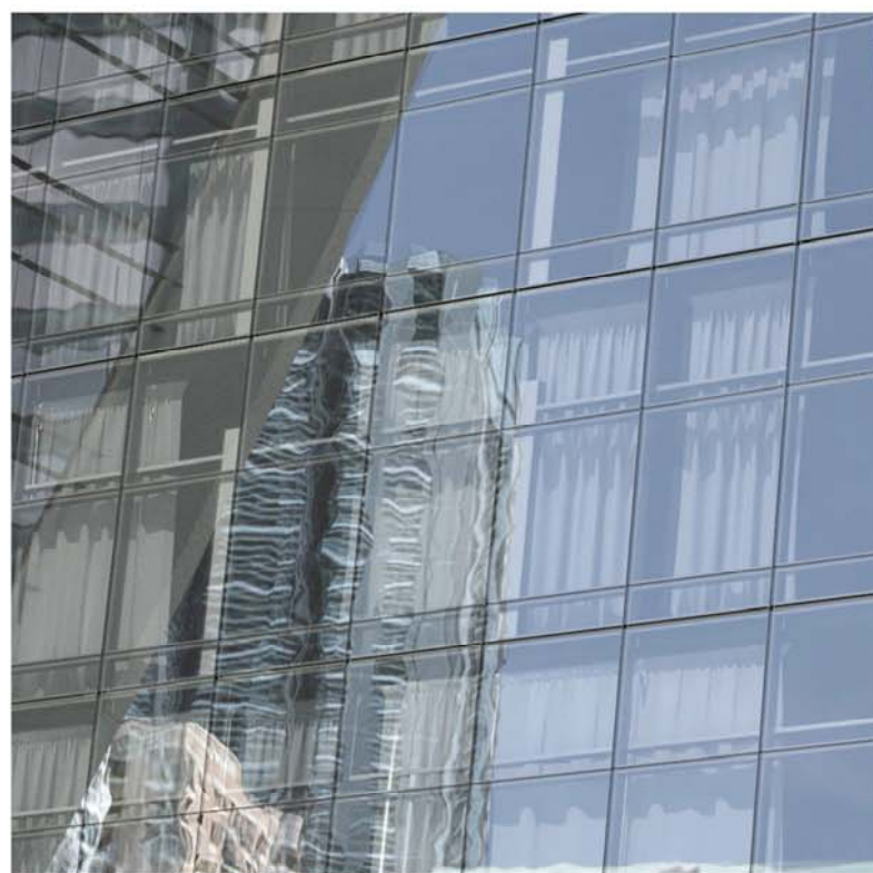
FT-3 Glazed curtain wall system with aluminium framing LOCATION: Recessed area of East Elevation
