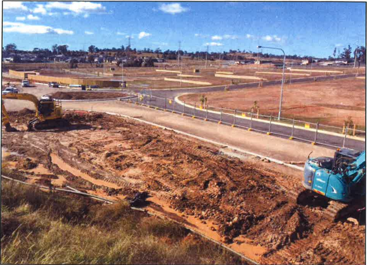
Figure 6: View of the site and residential dwellings opposite the site along The Hermitage Way taken from near the corner of The Hermitage Way and Digitaria Drive looking east (Source: Applicant's EIS)
