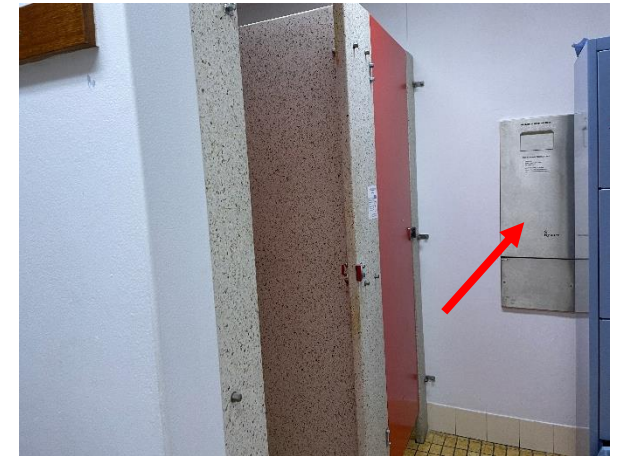
Photo 6: Main Warehouse – assumed internal asbestos containing insulation to incinerators within female toilets
