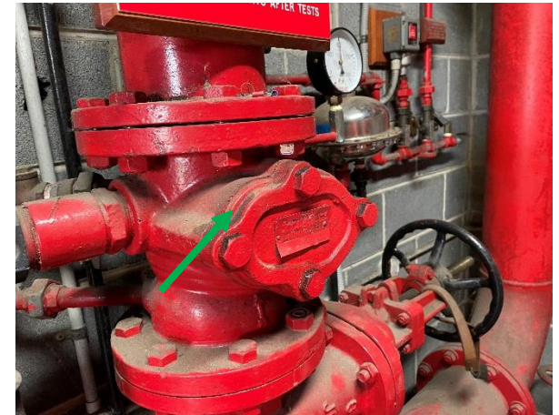
Photo 24: Water Storage Tank and Fire Booster Pump Shed – non-asbestos containing blue gasket to pump sprinkler valve
