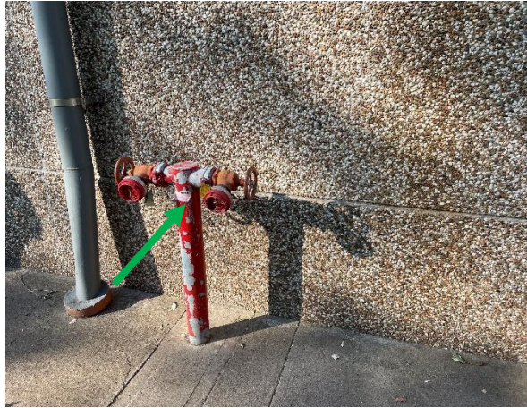
Photo 14: Main Warehouse – non-lead based red paint to the external fire hydrants
