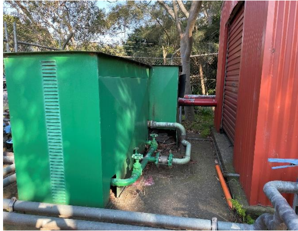
Photo 26: Overview of Hydrant Pump Room
