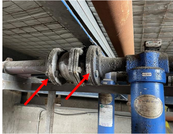
Photo 2: Main Warehouse – asbestos containing gaskets to redundant compressor pipework in central east portion, mezzanine level
