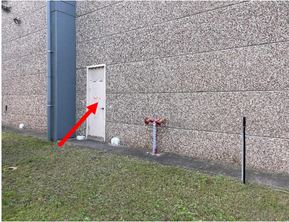
Photo 13: Main Warehouse – lead based beige paint to the external fire doors and frames
