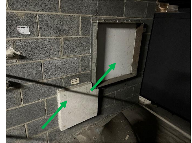
Photo 9: Main Warehouse – non-asbestos containing millboard to the wall penetrations within plant room 2 in central east portion
