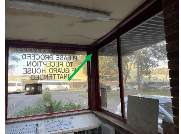
Photo 21: Gate House – lead based maroon paint to the internal and external steel framework
