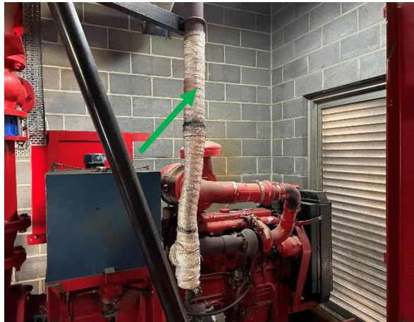
Photo 23: Water Storage Tank and Fire Booster Pump Shed – non-asbestos containing insulation wrap to exhaust pipe
