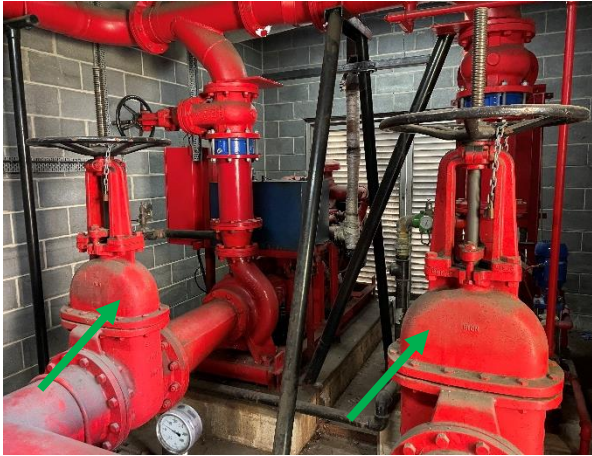
Photo 25: Water Storage Tank and Fire Booster Pump Shed – non-lead based red paint to hydrant pipework
