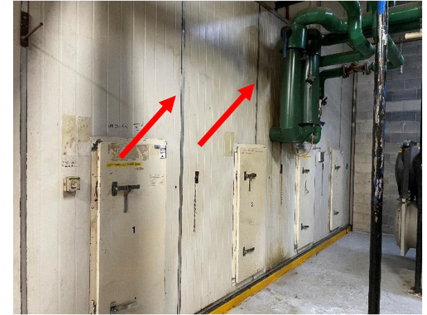
Photo 3: Main Warehouse – asbestos containing white mastic to the wall joins within the air handling units in central portion mezzanine plant room
