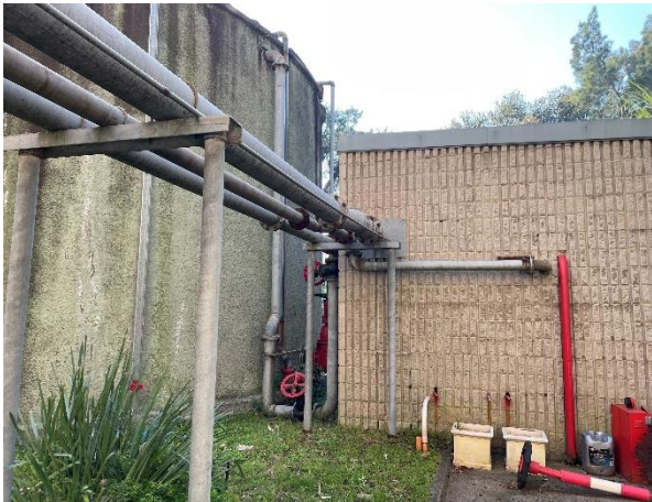
Photo 22: Overview of Water Storage Tank and Fire Booster Pump Shed
