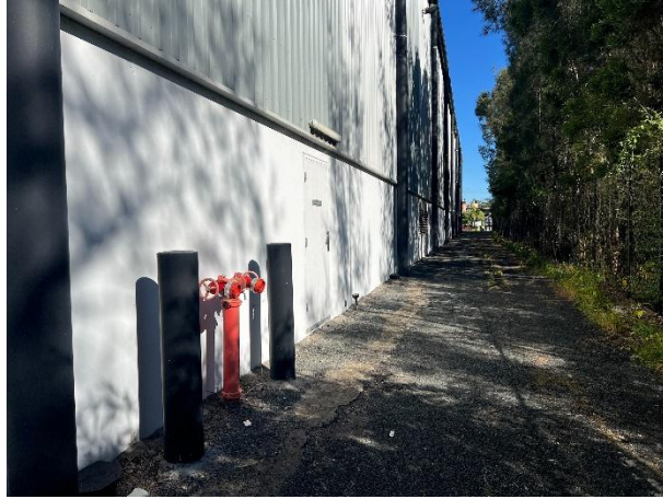
Existing Hydrant to north of building near northwest lot corner
