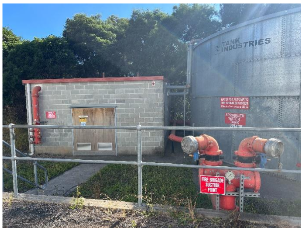
Existing Static Water Supply on site 550kL for sprinkler system
