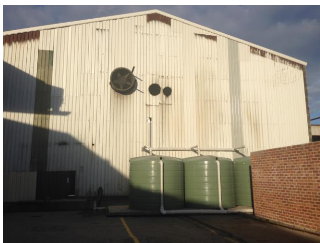
Figure 5-14 Rainwater storage tanks
