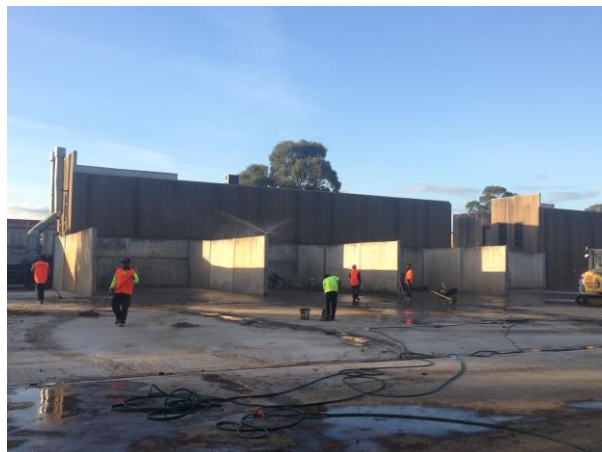
Figure 5-15 Water spray system for yard storage areas
