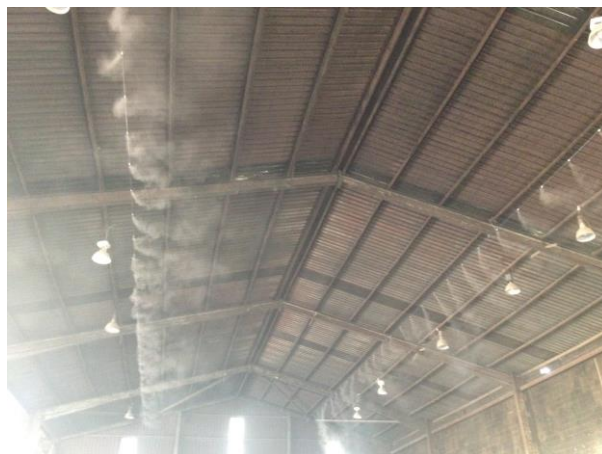
Figure 5-16 Fogging system for main processing building
