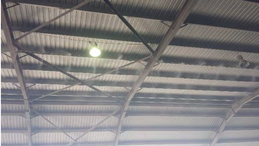
Photograph 9: Misting / fogging system in the materials processing warehouse
