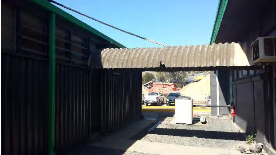
Photograph 3: Potential Asbestos Containing Material (PACM) roofing material along walkway between workshop and office building.
