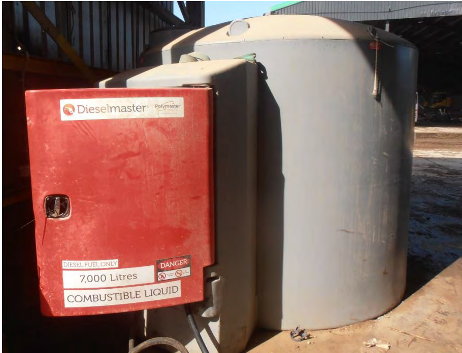
Photograph 1: 7000 L self bunded diesel AST located in the workshop.
