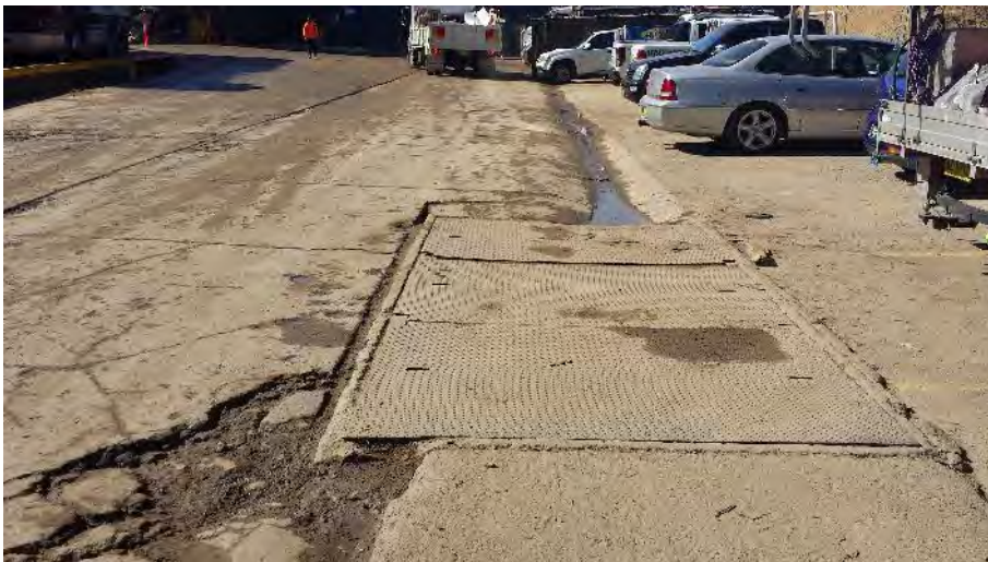
Photograph 10: Three stage sump pit located in the southern driveway. Central portion of the Site drains to this location prior to discharge to Council's stormwater network.
