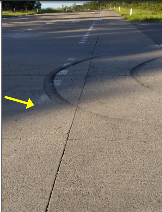
Photos 1 & 2: There is no intersection control for Italia Road at the highway (top photo), which is exacerbated by faded 'hold' line pavement marking (bottom photo). Moreover, the intersection sightboard on the far side of the highway is located beyond the crested section of highway making it less conspicuous, especially at night. Also, note the unprotected power pole within the clear zone on the left side of Italia Road approaching the highway junction (top photo).
