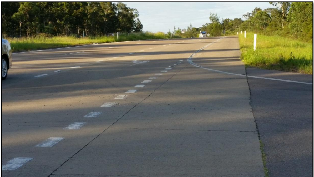
Photos 3 & 4: Safe intersection sight distance between the northbound highway travel lanes and the Italia Road junction is marginal (top photo – northbound highway approach to the Italia Road junction, bottom photo – looking south from the Italia Road junction). It is acknowledged that sight distance for truck drivers would be greater due to the higher driver position in the vehicle and that approaching northbound highway vehicles may be able to earlier sight trucks exiting the Italia Road junction due to the truck's larger (taller) size.
