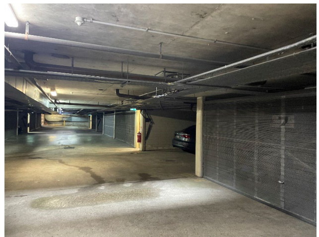
Figure 22 – view of the underground basement level, which extends from boundary to boundary.
