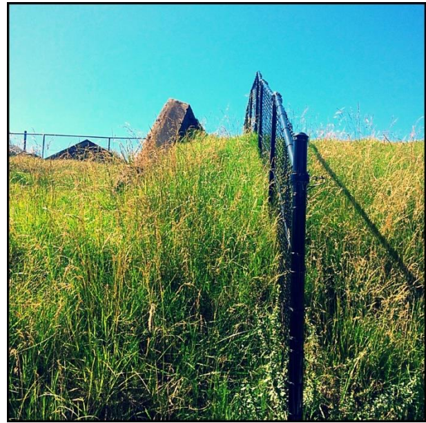
FIGURE 5: OVERGROWN GRASS, FOUNDRY WALL LOOKING NORTH
