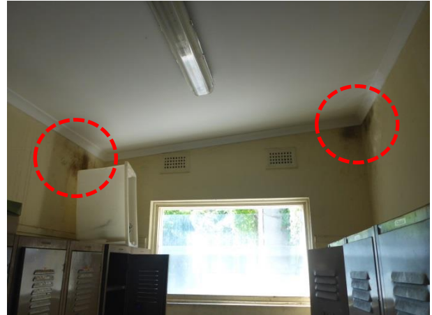
PICTURE 8 – VIEW OF A FORMER LOCKER ROOM, WITH MOULD GROWTH EVIDENT
