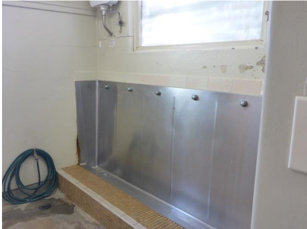
PICTURE 7 – VIEW OF THE MALE TOILETS (BLOCKED OFF FROM USE)
