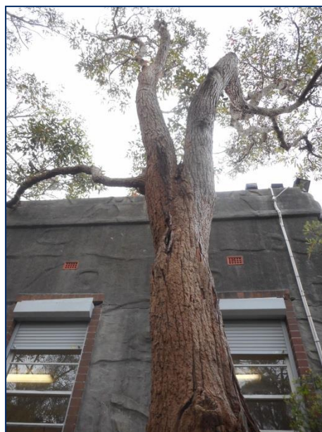
Figure 16 – The co-dominant structure of Tree 14, which has most of its canopy positioned above the adjacent structure, probably due to phototropic growth towards the north. Recommended for removal.
