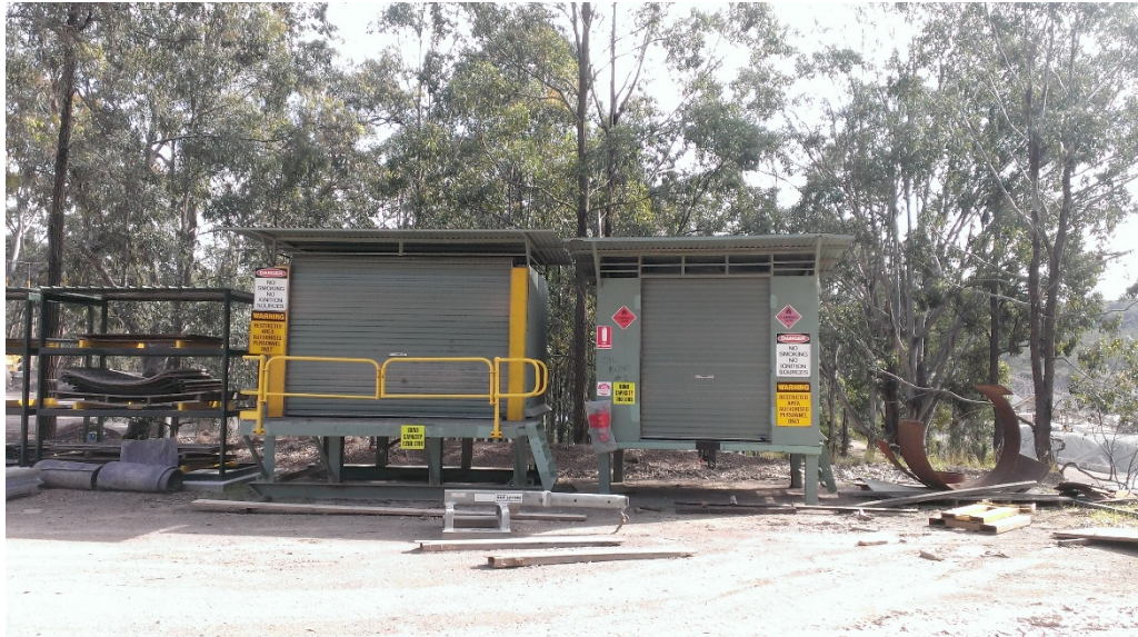
Photograph 15-3 Typical Lubricant and hydraulic oil storage standard used by Hanson.
