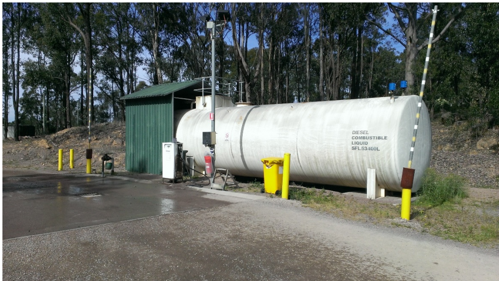
Photograph 15-2 Typical Self-bunded Diesel storage.
