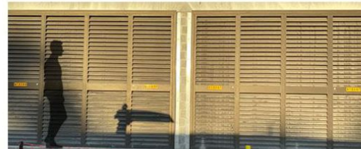
Ventilation louvres on the front of a chamber substation
